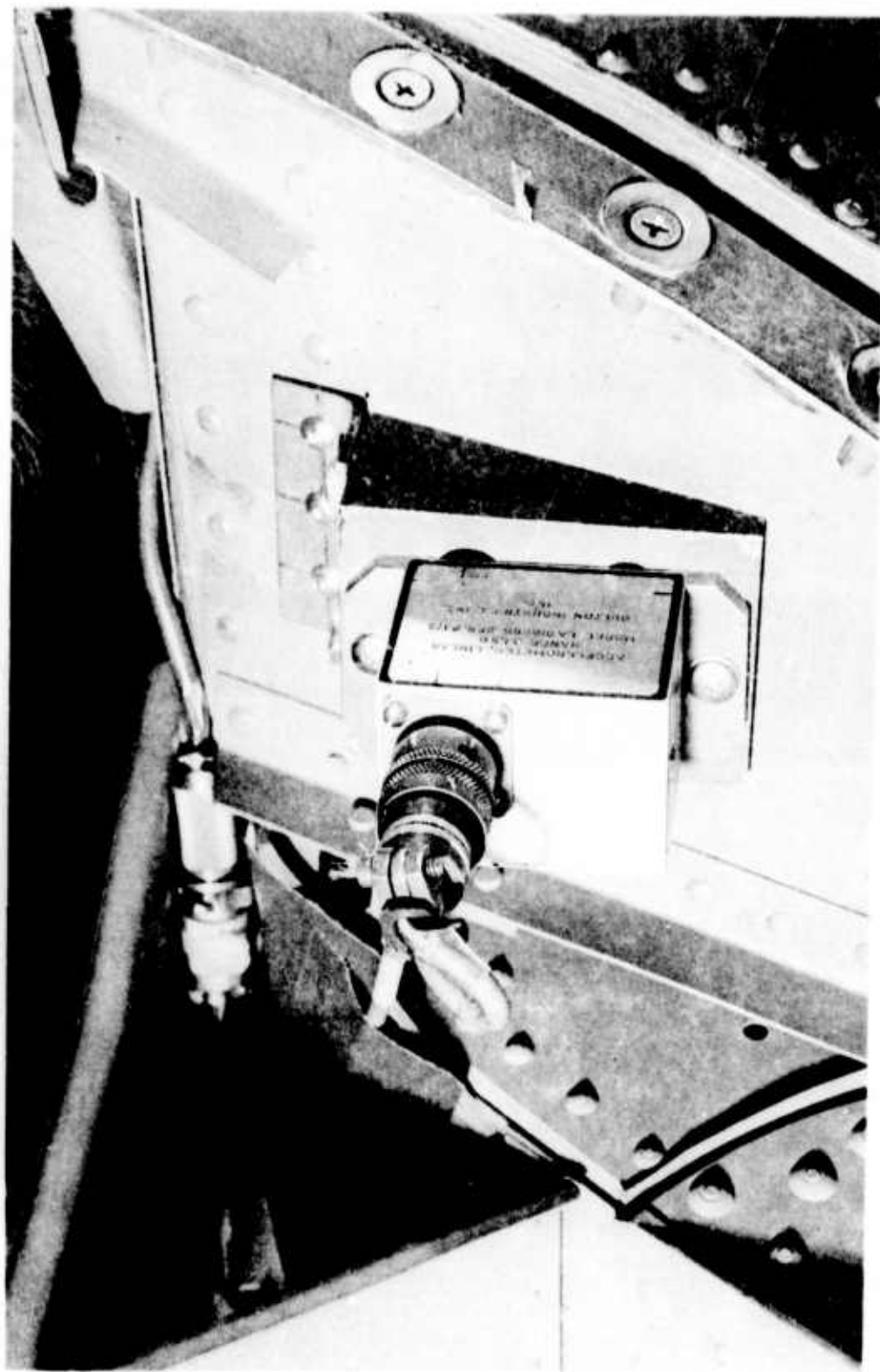
Photo 8. Vertical Accelerometer Installation FS 50 Left
