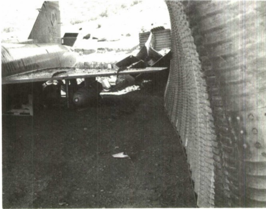
Figure 12. Displacement of Wall in Shelter A
