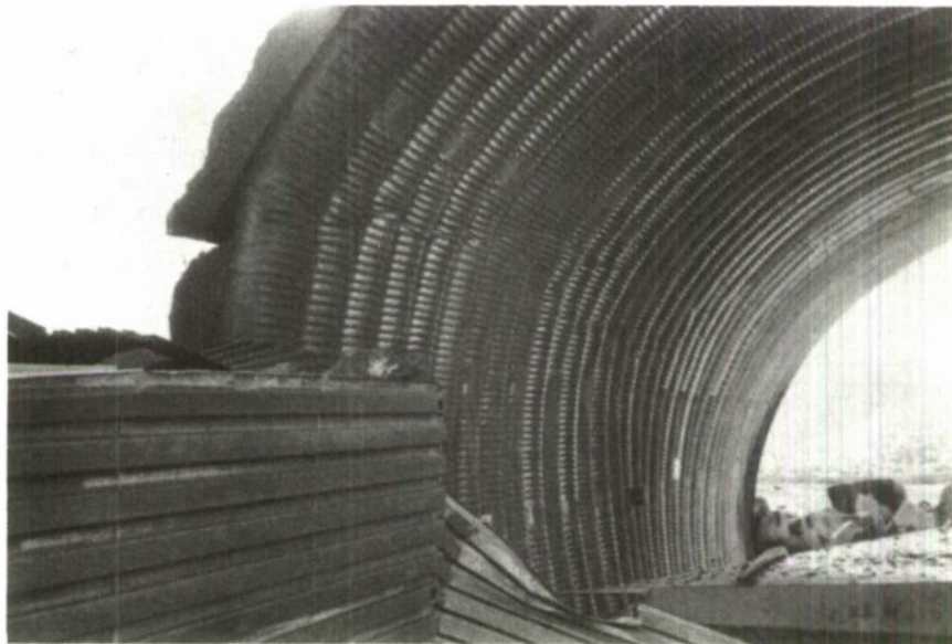
Figure 13. Hinging of Acceptor Wall (Shelter A)
