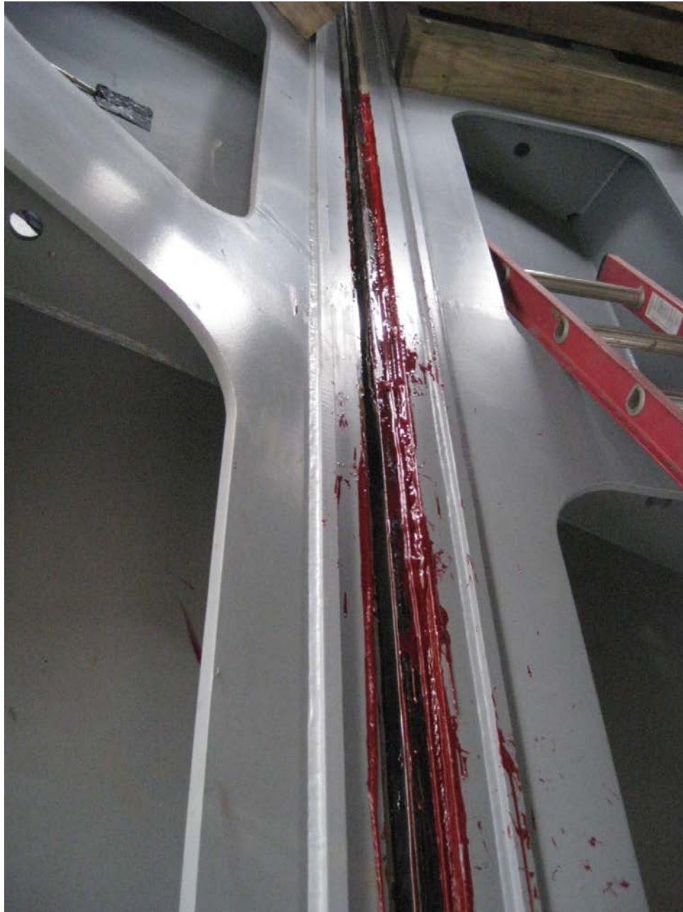
Figure 2-3. Backing material blowouts and leakage.
