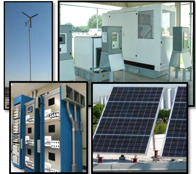
Microgrid Development Center
