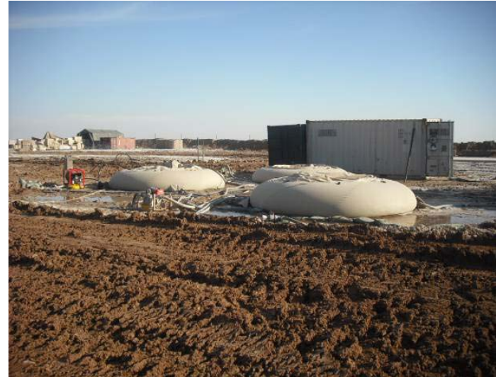
Potable Water Available (Concern is Distribution)
