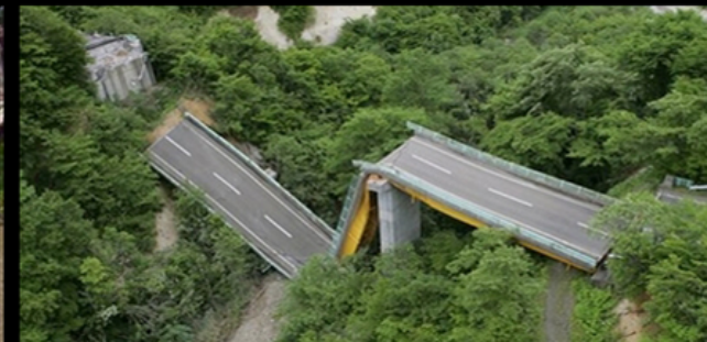
Earthquake – NE Japan
