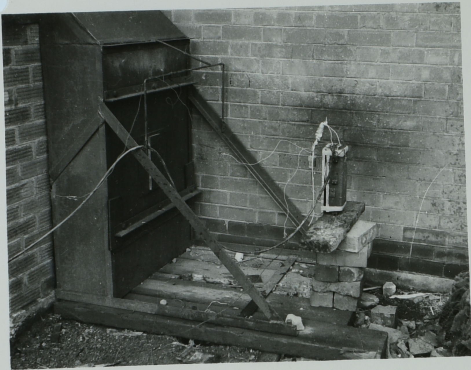
Photograph showing steel screen for protection of X-ray tube and charge and cassette in position.
