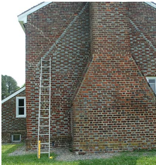
Matthew Jones House crack at Northwest Photo credit: Michael C. Henry
