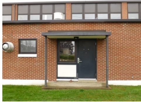
Replacement anodized-bronze aluminum single-pane window with fiberglass panel below, replacement metal entry door, and flat roof canopy the west elevation (ERDC-CERL, 2014).
