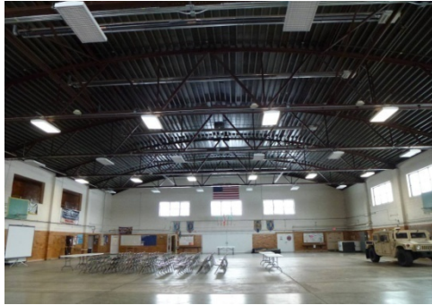
Interior view of the double-height drill hall space with concrete floor, concrete and glazed sanitary tile walls, barrel roof with exposed arched truss system (ERDC-CERL, 2014).
