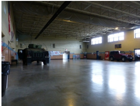
Interior view of the open drill hall, concrete floor, clerestory windows, concrete-block and glazed sanitary tile walls, and truss roofing system (ERDC-CERL, 2013).
