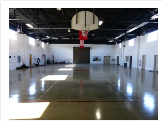
Interior view of the open double-height drill hall with concrete floor, combination of concrete-block and glazed sanitary tile walls, clerestory windows, and exposed truss roof system (ERDC-CERL, 2014).
