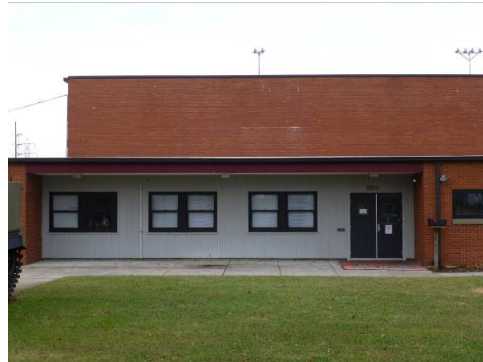
Entry bay on the east (front) elevation with original wood paneled wall, replacement one-over-one anodized-bronze aluminum paired windows, and paired replacement metal entry doors (ERDC-CERL, 2013).
