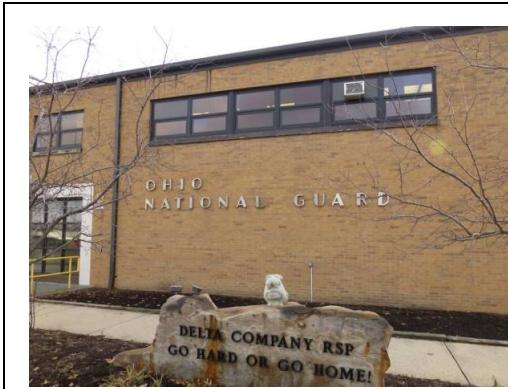
Original ribbon-style window opening with replacement one-over-one anodized-bronze aluminum windows and original Stainless-steel lettering (ERDC-CERL, 2013).
