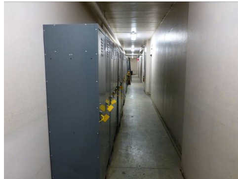
Looking down the corridor in the basement, with the original rifle range on the right side of the hall (ERDC-CERL, 2013).
