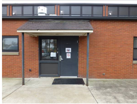
Replacement anodized-bronze aluminum single-pane window with fiberglass panel below, replacement metal entry door, and modified flat roof canopy on the north elevation (ERDC-CERL, 2013).
