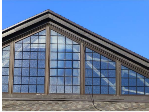
Triangular window in the gable end of the riding stadium roof (ERDC-CERL, 2013).
