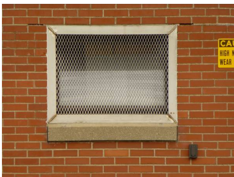
Original small single window opening with replacement anodized-bronze aluminum window with metal mesh screen cover (ERDC-CERL, 2013).
