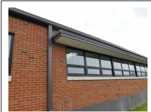
Original ribbon-style window opening and concrete sunshade canopy above with replacement anodized-bronze aluminum windows (ERDC-CERL, 2013).
