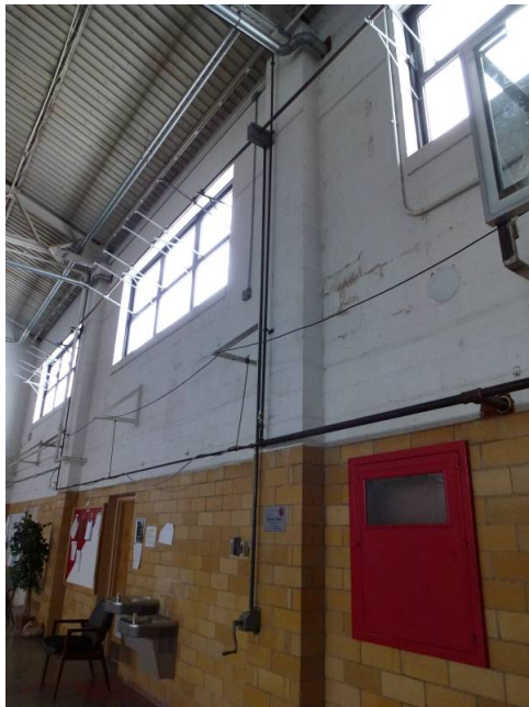
Glazed sanitary tile wall and clerestory windows in the drill hall space (ERDC-CERL, 2014).
