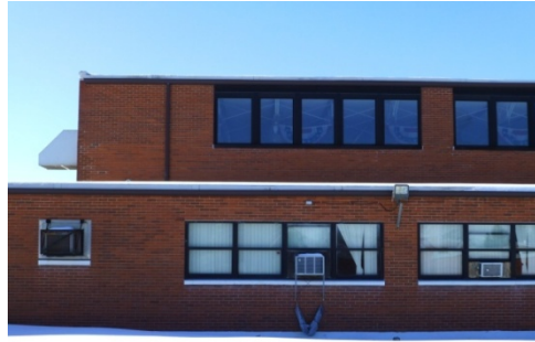
Original group window openings and clerestory window openings with replacement anodized-bronze aluminum window (ERDC-CERL, 2014).
