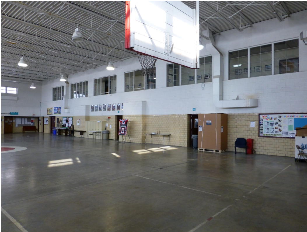
Figure 58. Interior view of the drill hall, looking at interior windows of the second-floor corridor of Springfield OHARNG Armory (ERDC-CERL, 2014).
