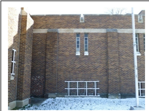
Narrow window openings [metal-sash windows are noncontributing] (St. Marys OHARNG Armory, ERDC-CERL, 2013).
