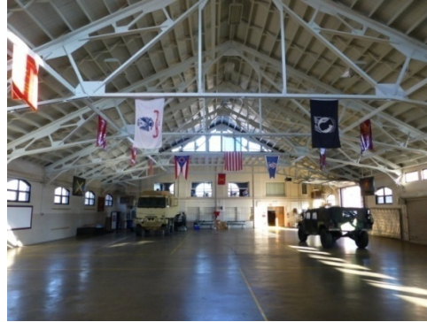
Interior view of the open riding stadium space with exposed wood rafters and steel truss roofing system (ERDC-CERL, 2013).
