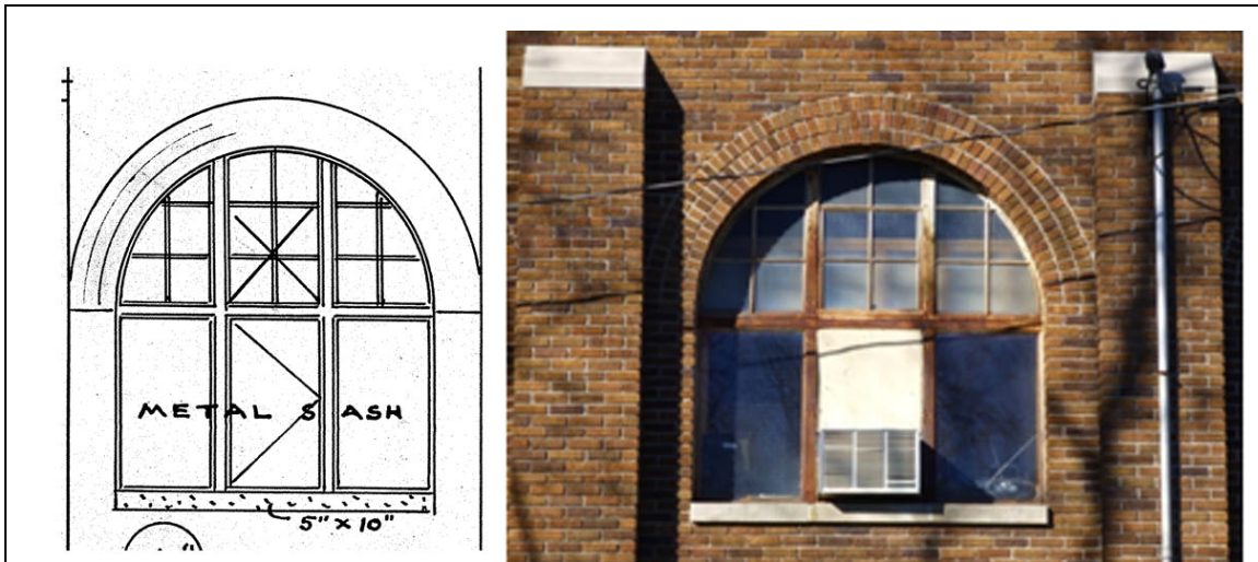
Windows on the southeast (rear) elevation of the 1938 addition: original design and materials with metal frame with wire glass, brick lintels, and stone windowsills on the left (drawing), compared to the current condition of the modified window openings on the right (ERDC-CERL, 2013).
