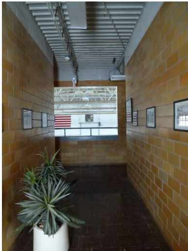
Second floor corridor with glazed sanitary tile walls and exposed roofing system for the ceiling (ERDC-CERL, 2014).
