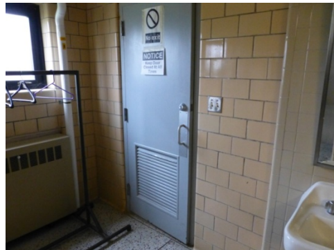
Original glazed sanitary tile walls of the latrine and original metal door leading from men's latrine into the adjacent locker room (ERDC-CERL, 2013).
