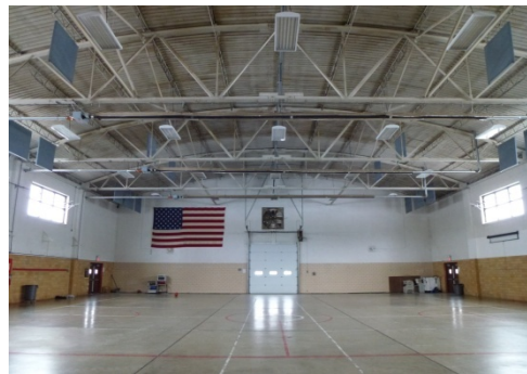
Interior view of the open drill hall space with concrete floor, glazed sanitary tile walls, barrel roof, and expose arched steel truss roofing system (ERDC-CERL, 2014).
