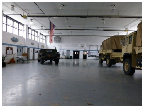
Interior view of the open drill hall, concrete floor, clerestory windows, concrete-block walls, and steel I-beam roofing system (ERDC-CERL, 2013).
