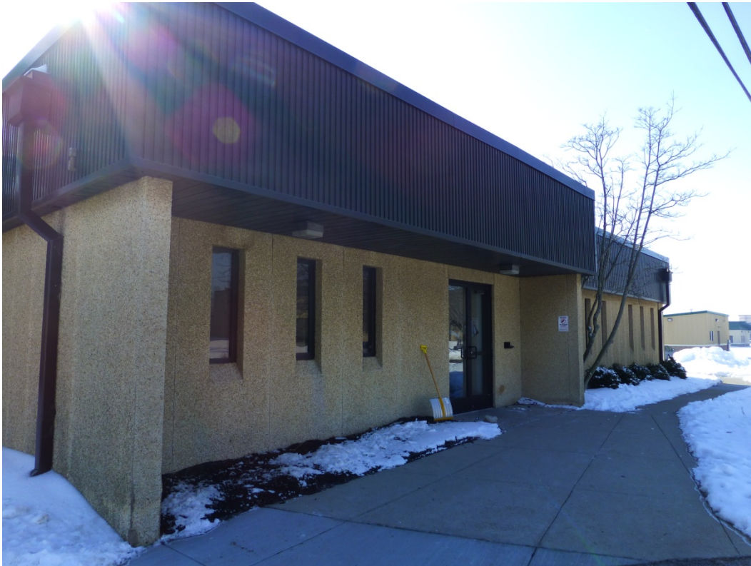
Figure 86. Modified main entry with new window pattern, new windows, new doors, new exterior wall cladding material, and new metal fascia system (ERDC-CERL, 2014).
