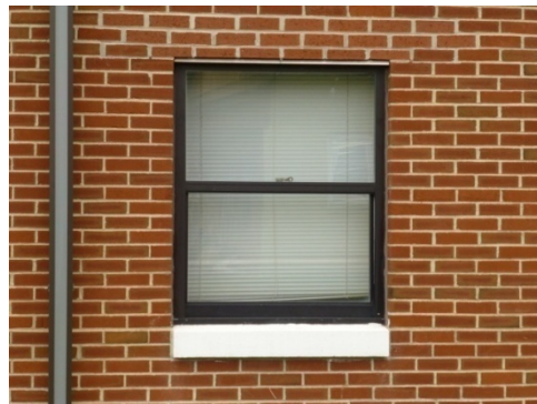
Original single window opening with replacement anodized-bronze aluminum one-over-one window on the right side of the west elevation (ERDC-CERL, 2013).
