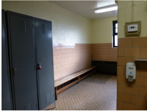
Glazed sanitary tile walls and mosaic tile floor in the latrines (ERDC-CERL, 2013).
