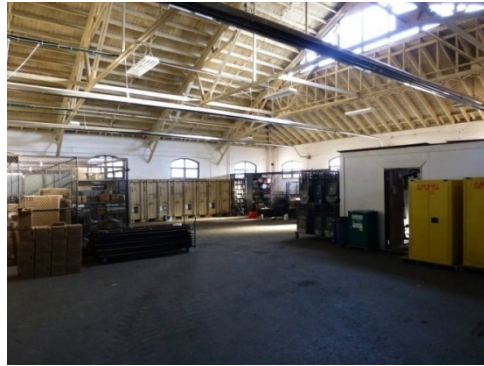
Interior view of the open riding stadium with exposed wood rafters and steel truss roofing system (ERDC-CERL, 2013).
