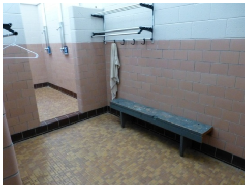
Glazed sanitary tile walls and mosaic tile floor in the latrines (ERDC-CERL, 2013).
