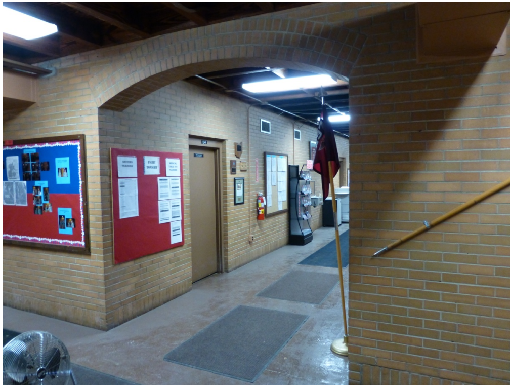
Figure 27. Arched brick passageways in corridors on the first floor of the Akron-Hawkins OHARNG Armory (ERDC-CERL, 2013).
