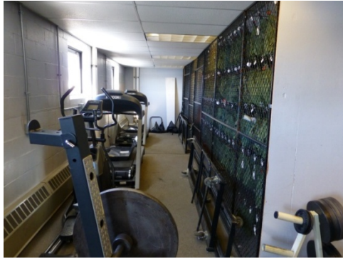
Interior view of the modified space of the original rifle range now used for storage/weight room/offices (ERDC-CERL, 2014).
