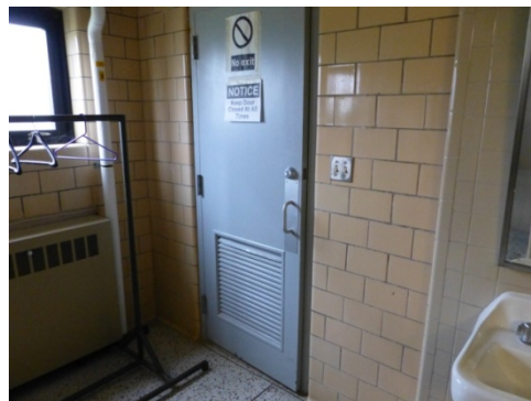
Original glazed sanitary tile walls of the latrine and original metal door leading from men's latrine into the adjacent locker room (ERDC-CERL, 2013).
