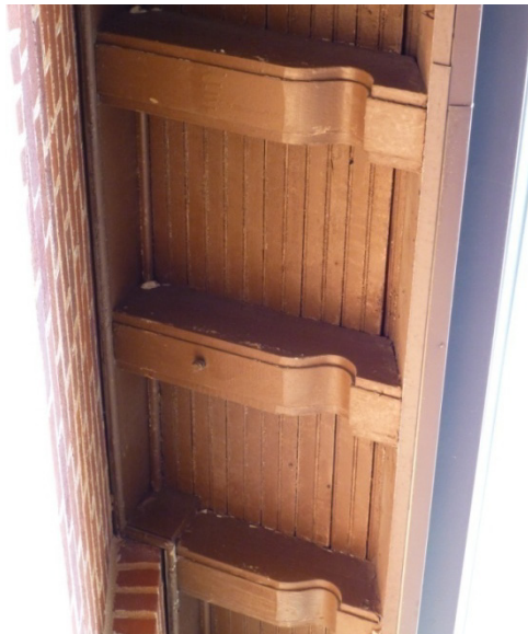
Decorative wood rafters and overhanging eave of the roof over the riding stadium (ERDC-CERL, 2013).
