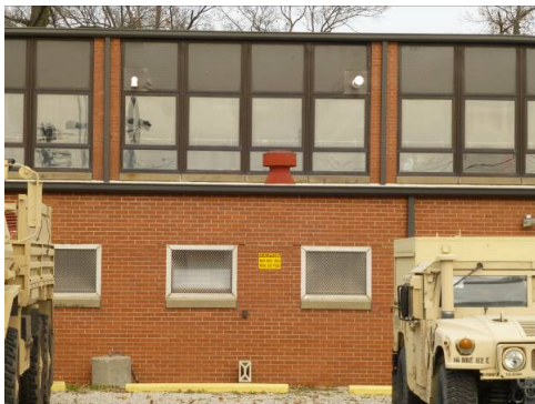
Original clerestory window openings with replacement anodized-bronze aluminum windows with fiberglass panel inserts (ERDC-CERL, 2013).
