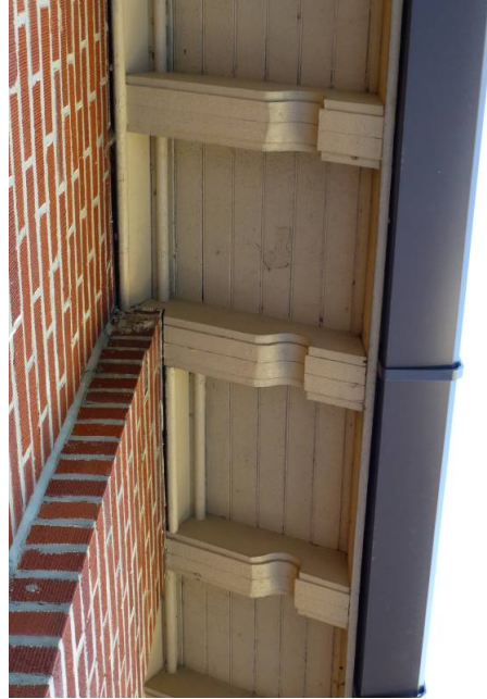
Decorative wood rafters and overhanging eave of the riding stadium roof (ERDC-CERL, 2013).
