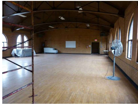
Interior view of open assembly hall with wood floor, brick wall, barrel roof, and arched steel truss roof system (ERDC-CERL, 2013).
