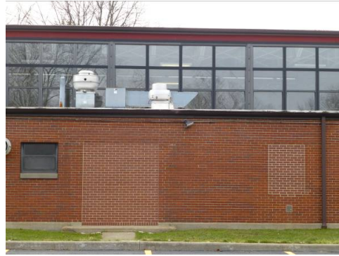
Modified single door opening with sidelight and flat roof canopy, opening filled with brick on the north elevation (ERDC-CERL, 2013).
