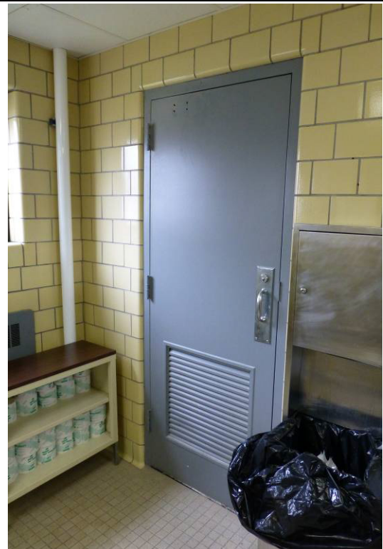
Original glazed sanitary tile walls of the latrine and original metal door leading from men's latrine into the adjacent locker room (ERDC-CERL, 2013).
