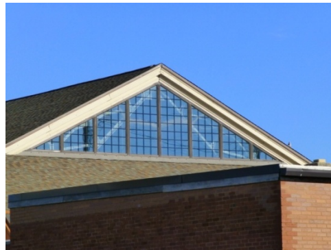
Triangular window in the gable end of the roof over the riding stadium (ERDC-CERL, 2013).
