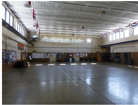
Interior view of the open drill hall, concrete floor, clerestory windows, concrete-block and glazed sanitary tile walls, and truss roofing system (ERDC-CERL, 2014).
