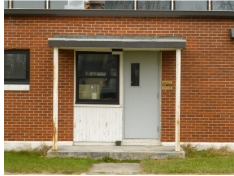
Replacement anodized-bronze aluminum single-pane window with fiberglass panel below, replacement metal entry door, and flat roof canopy on the south elevation (ERDC-CERL, 2013).
