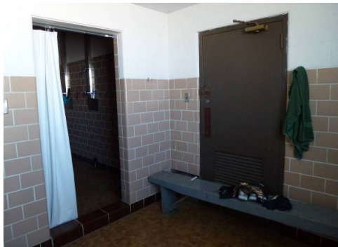
Glazed sanitary tile walls in the latrines and original metal door leading to the old locker room (ERDC-CERL, 2014).
