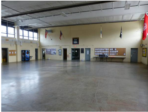
Interior view of the open drill hall, concrete floor, clerestory windows, concrete-block walls, and steel I-beam roofing system (ERDC-CERL, 2013).
