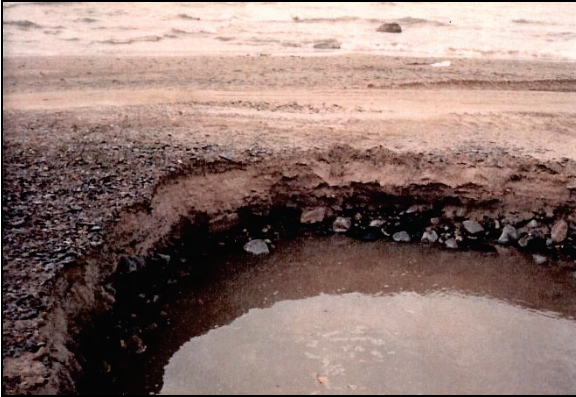
Figure 86. Excavation in west fillet at Sturgeon Point pre-project construction (16 Nov 1988). Photograph shows high quantity of shale plates in soil column (USACE 2004).
