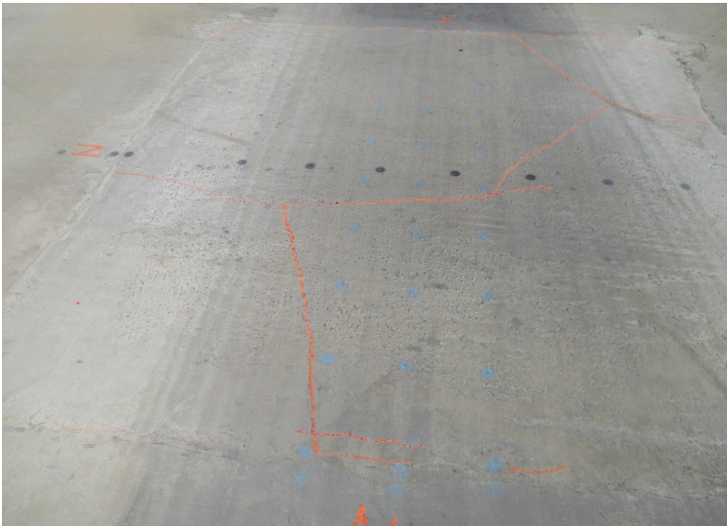
Figure 28. Series 3, Repair 10-1 - low-severity shattered slab at 560 passes.
