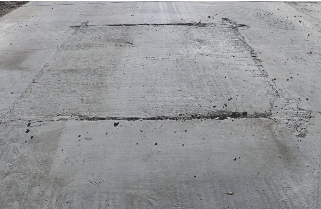
Figure 22. Series 1, Repair 3 - overall at failure (3,000 passes).
