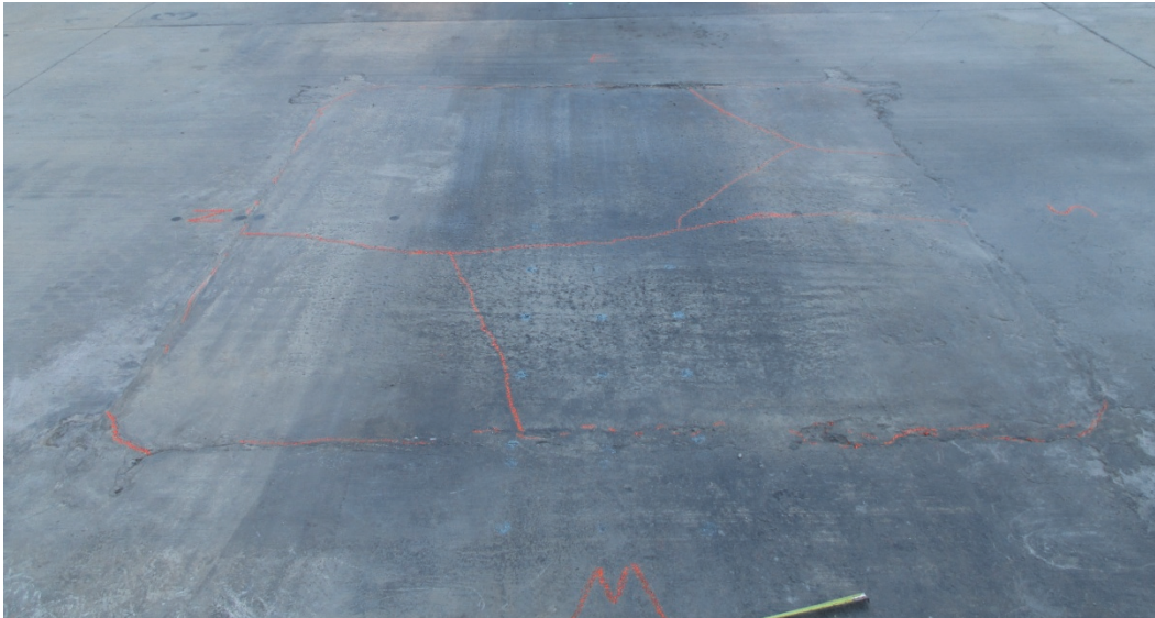
Figure 29. Series 3, Repair 10-1 - not failed at 10,000 passes.
