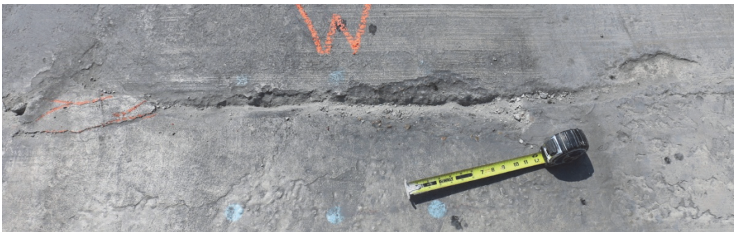
Figure 27. Series 3, Repair 9 - west edge at failure (3,500 passes).
