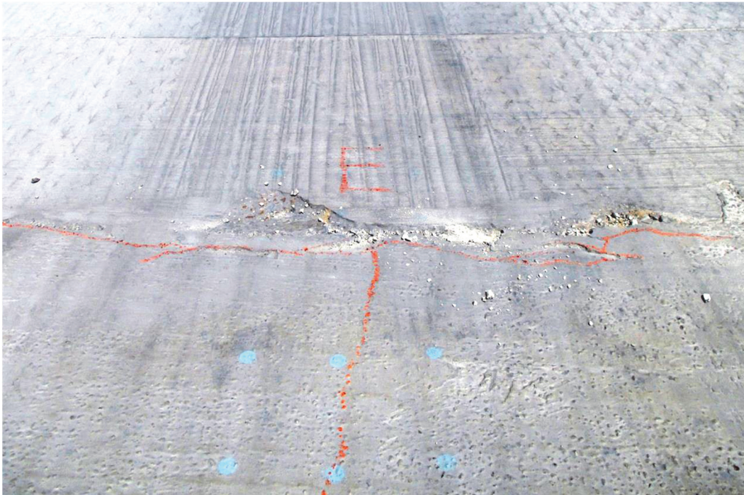
Figure 25. Series 2, Repair 7-1 - overall at failure (2,500 passes).
