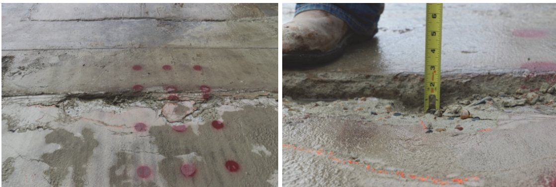
Figure 20. Series 1, Repair 1 - west edge at failure (560 passes).
