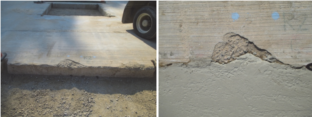
Figure 24. Spalled parent PCC for Series 2, Repair 7-1 - spalled areas on east edge (left) and partially filled spall prior to traffic (right).
