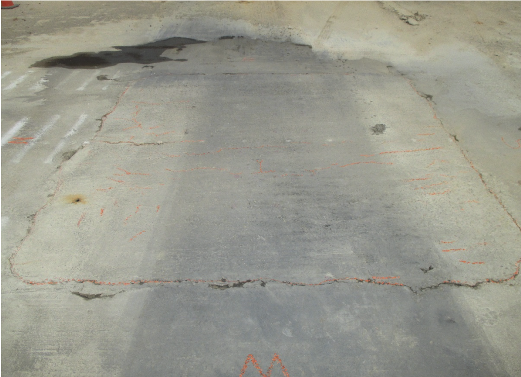
Figure 31. Series 4, Repair 14 - after 10,000 passes.
