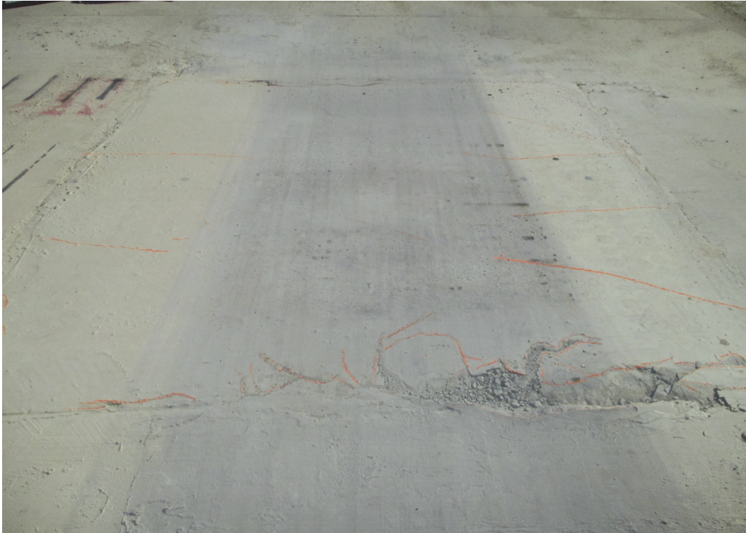
Figure 33. Repair 15 at failure of 1,508 passes.
