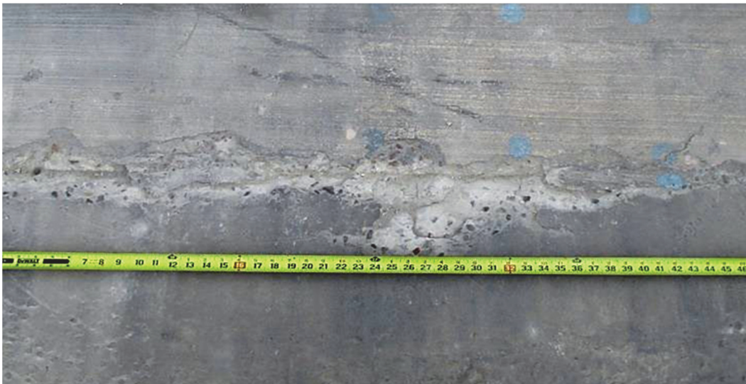
Figure 23. Series 2, Repair 6 - east edge at failure (1,300 passes).
