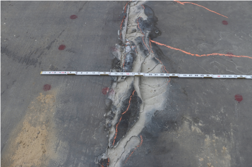
Figure 7. Joint spall presenting high FOD (swept) and tire damage potential.
