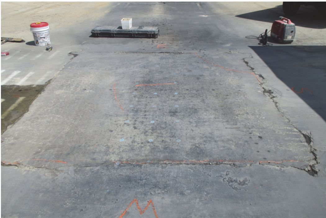
Figure 30. Series 3, Repair 11 - not failed at 10,000 passes.
