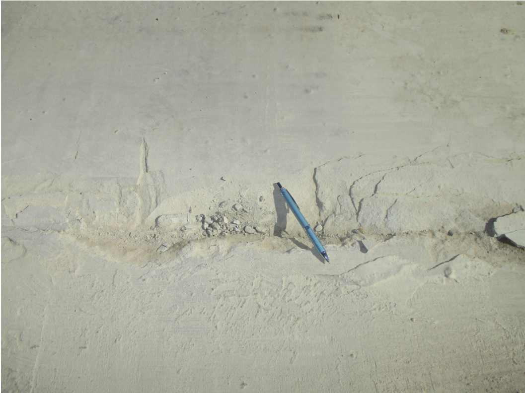
Figure 32. Repair 15 spalling at 800 passes (after being swept).
