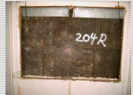
Rear side of concrete inside the container
