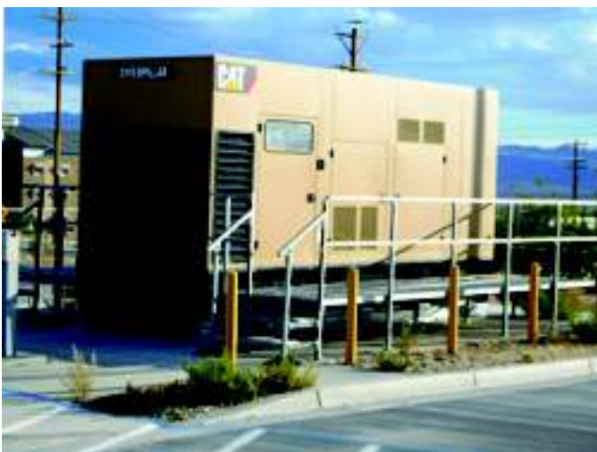
Diesel backup generator
