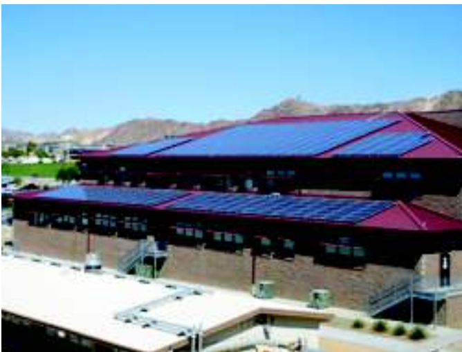
Building-mounted PV Solar Array
