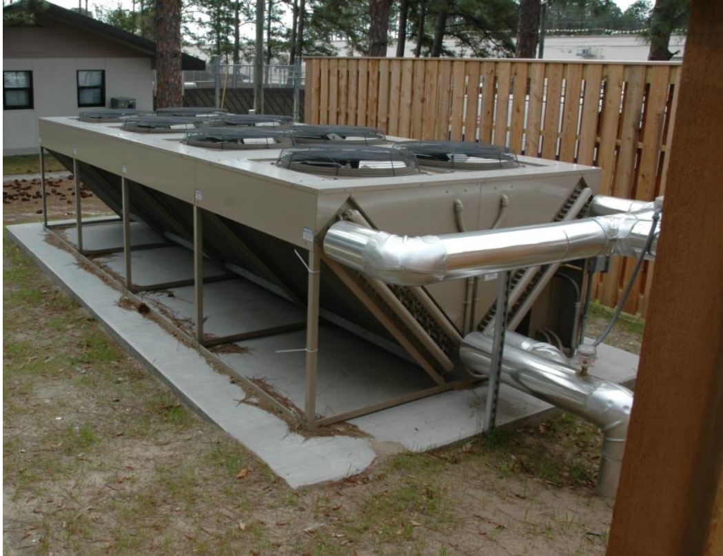
Figure 5.12. Dry fluid cooler installed at Building 584.
