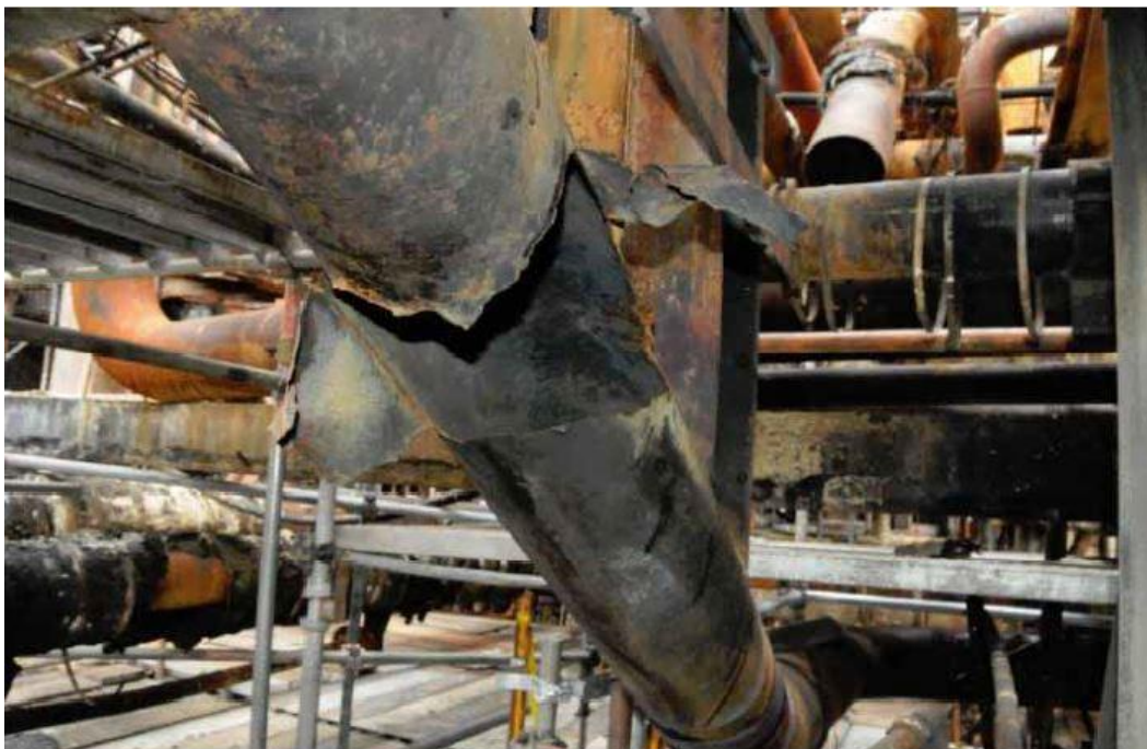
Figure 11. Photo of Ruptured Process Line
