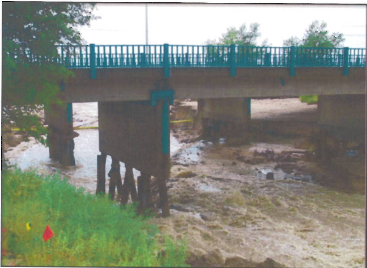
Figure 2. Platte Avenue over Sand Creek, Colorado Springs, 2009 Courtesy City of Colorado Springs
