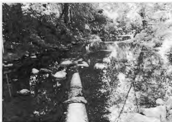
Figure 19. Picture at Site F depicting the exposed concrete sewer pipe (bottom center)
