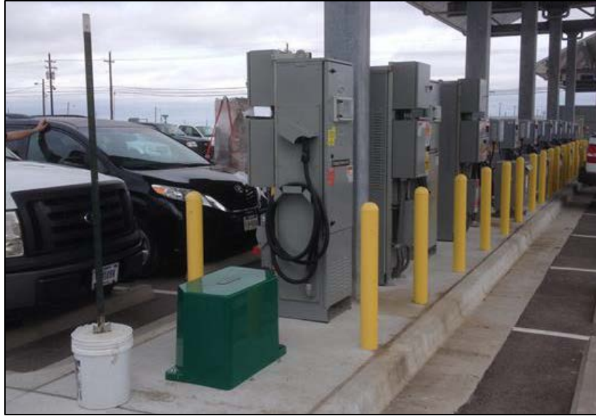
Figure 20. Fort Hood EV Lot
