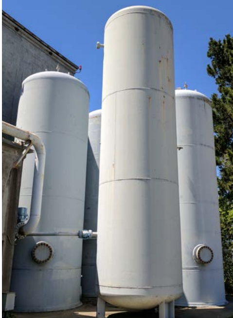
Figure 16. Air Storage Tanks at NPS IMPEL
