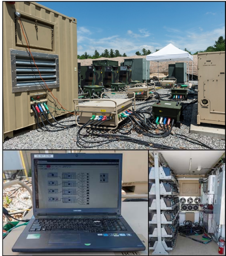
Figure 34: Energy Informed Operations-Central
