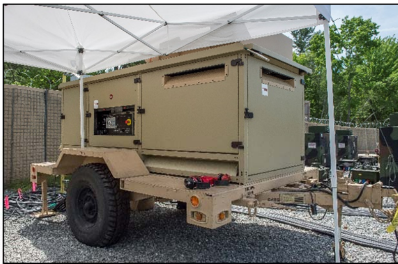
Figure 30: T100 Genset on Trailer
