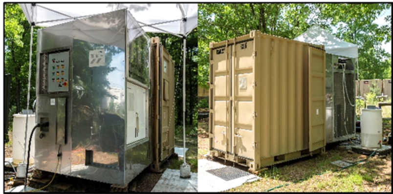
Figure 73: Containerized Ice Making Technologies
