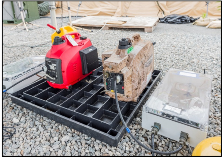
Figure 39: Man-Portable Genset for Power Generation
