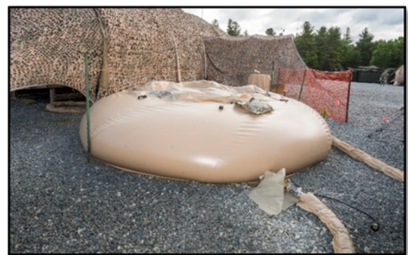
Figure 52: 3000-gal Graywater Tank
