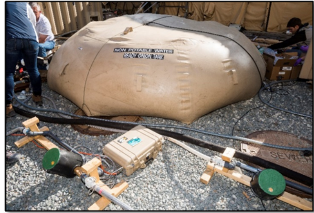
Figure 53: 3000-gal Non-potable Water Tank
