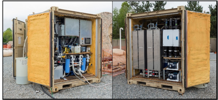
Figure 50: Graywater Reuse System – Forward Osmosis/Reverse Osmosis
