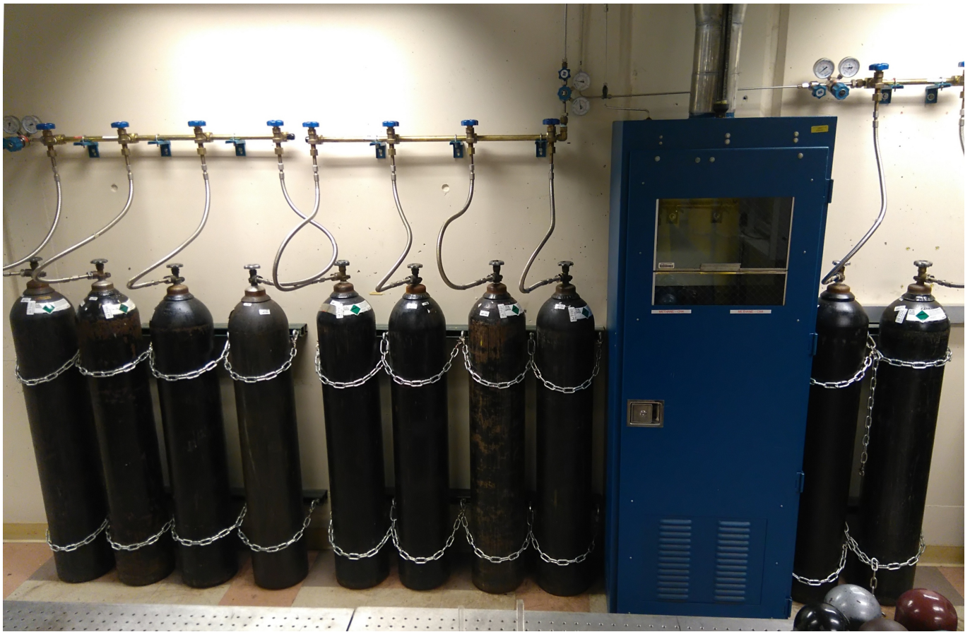
Figure 4: Photo showing 10 nitrogen gas cylinders attached to two quadrupole manifolds and one double manifold. Two cylinders that supply gaseous fuel are placed in the cabinet.
