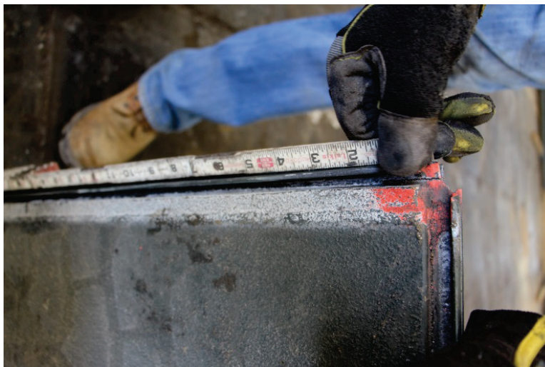
Figure 5.6. 4 in. crack in upper rail of underlap connector on panel 54.
