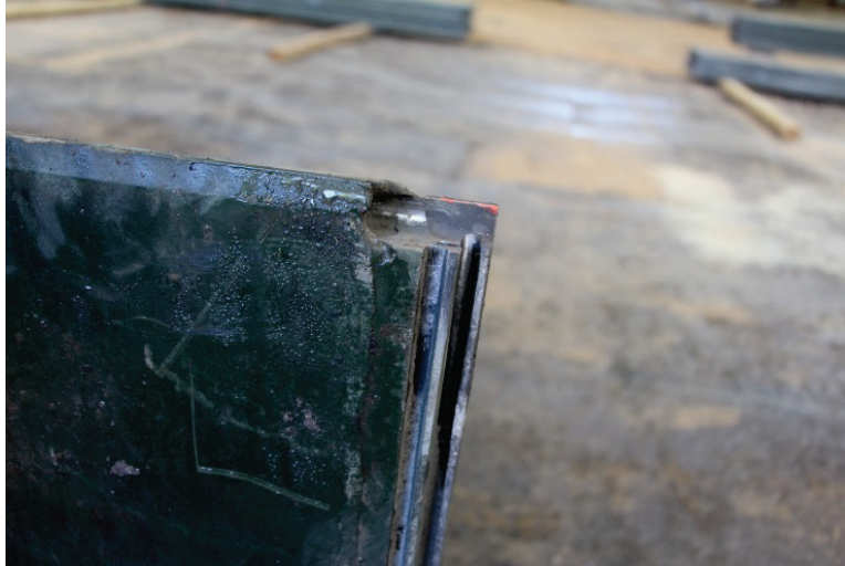
Figure 5.7. 1 in. crack on upper rail of underlap connector on panel 102.
