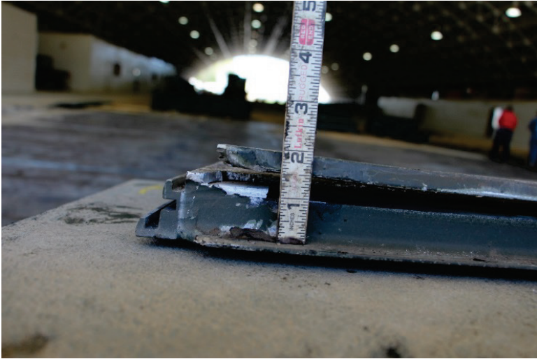
Figure 5.2. Female hinge crack in panel 3.
