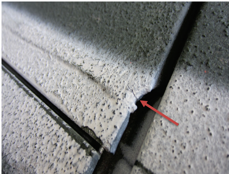
Figure 4.1. Hairline crack in panel 74 observed after pass 1,008.
