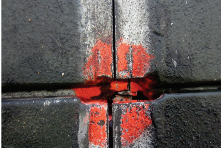
Figure 5.5. Top skin tear in upper rail of overlap connector on panel 53.
