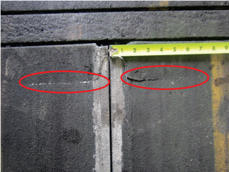
Figure 4.4. Cracks propagating in panels 2 and 3 at pass 6,100.
