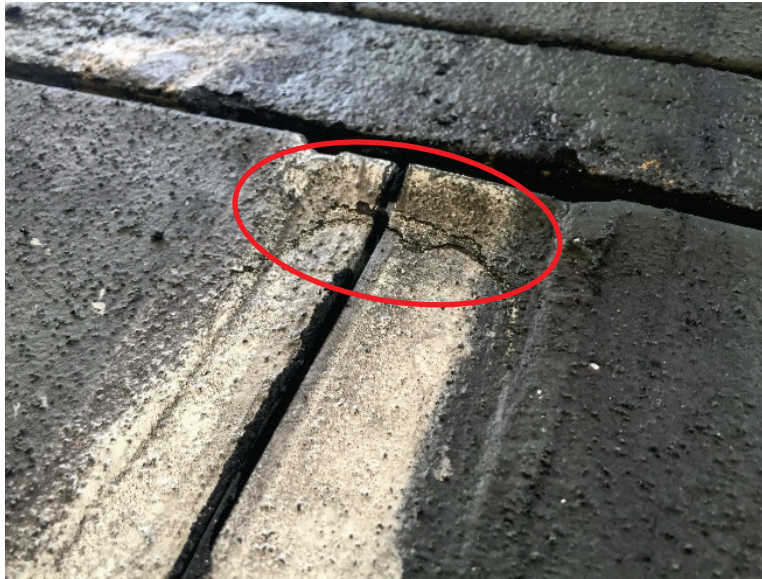
Figure 4.2. Corner curl cracks in panels 2 and 3 at 4,576 passes.
