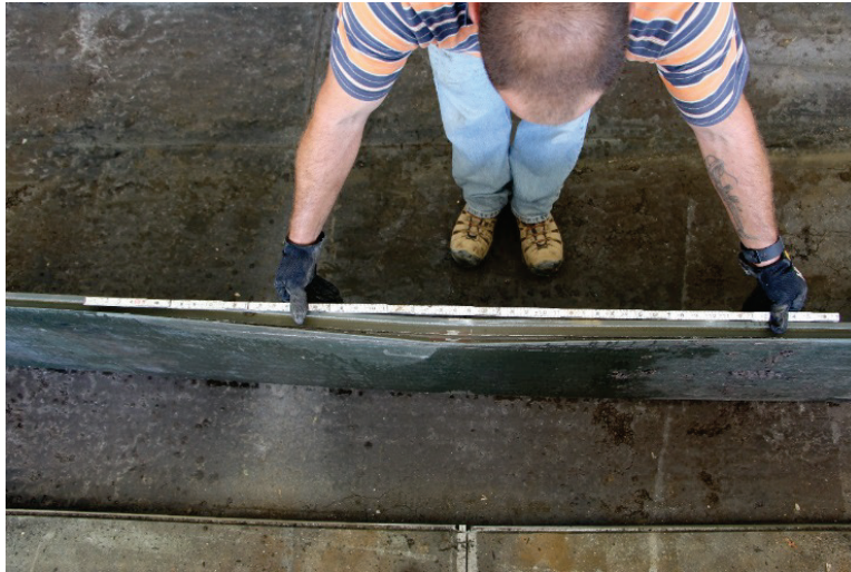
Figure 5.3. 54 in. female hinge connector crack on panel 8.
