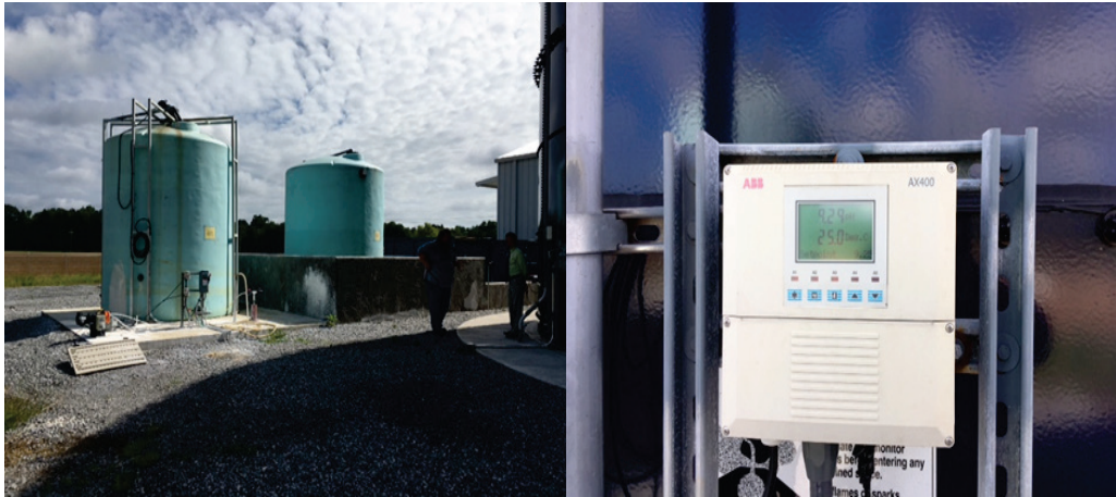
Figure 5. Lime slurry tank and pH meter on equalization tank.
