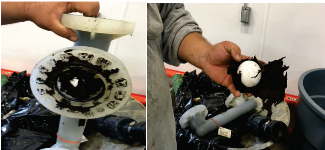
Figure 12. Clogging of the ball check valve in the pneumatic sludge pump.
