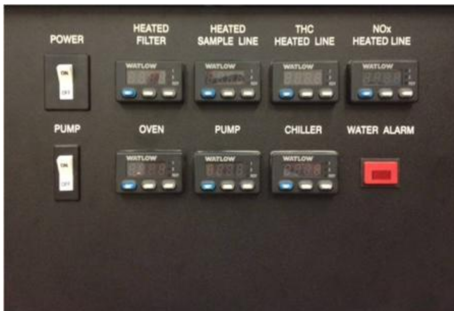
Figure A.2: CAI power and diagnostics panel [56]
