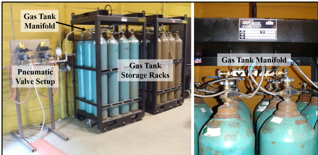
Figure 3. Gas management system (left) and close up of the gas manifold (right).
