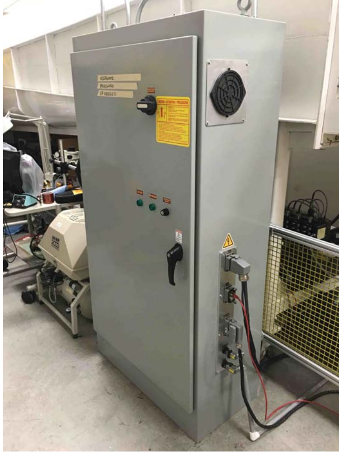
Figure 11. MTA Computer Assembly Cabinet
