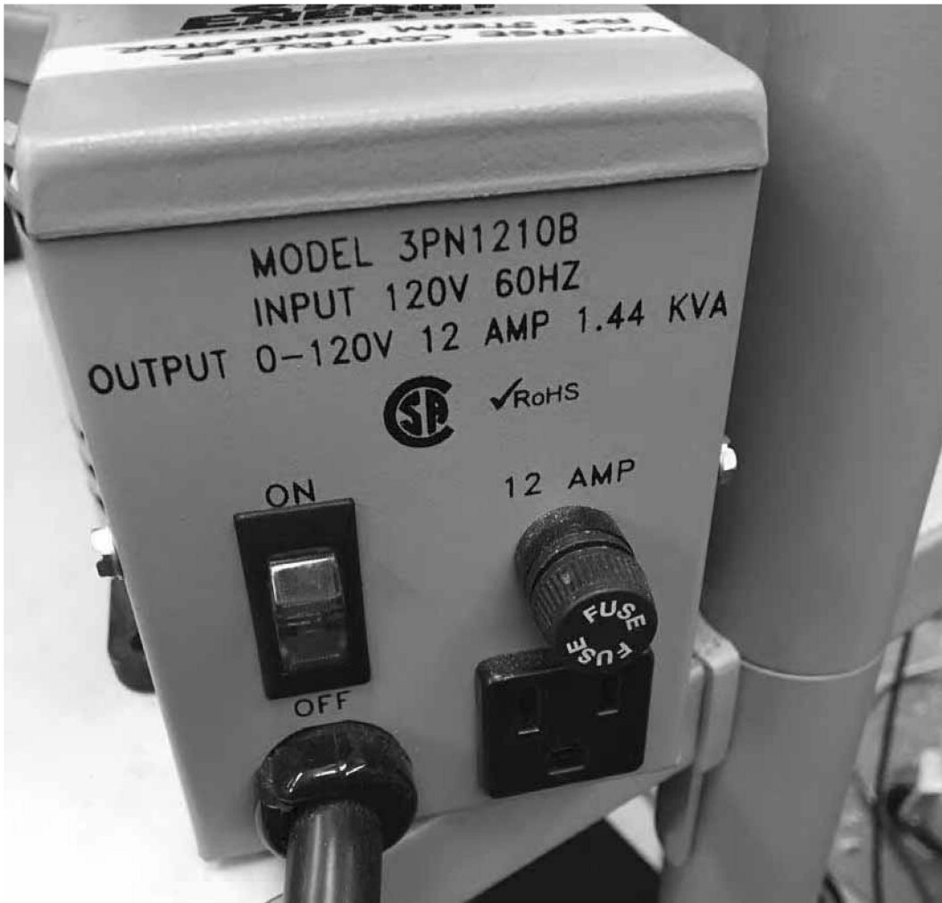
Figure 48. Voltage controller for steam generator. Steam generator power is controlled using the switch on the left side
