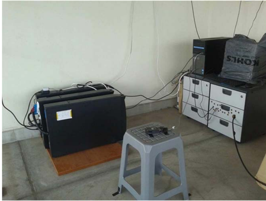
Figure 1-10 Receiver System at Nanyang House, which includes uninterrupted power supply and magnetometer.
