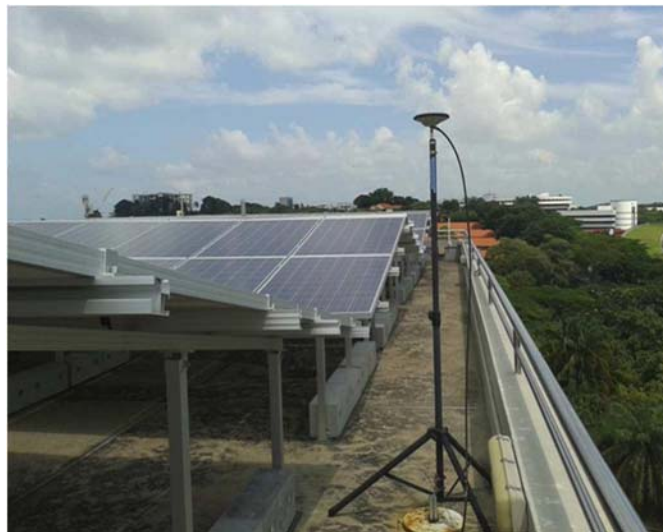
Figure 1-11: Multi Frequency GNSS Antenna at Nanyang House
