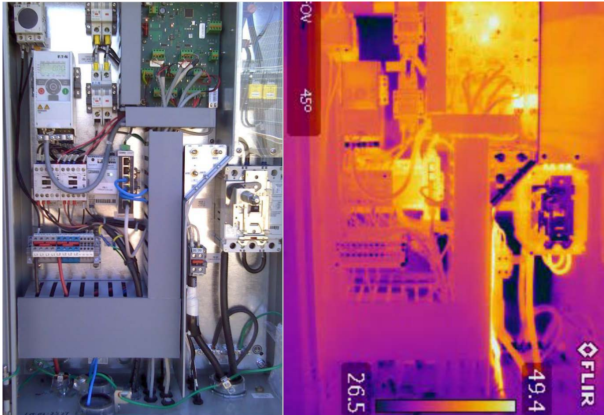
Figure 8. (Left) The internal visible image of one of the tracker control boxes. On the lower right of the image two large black wires are seen exiting the enclosure. These wires are the current carrying conductors that lead to system combiner boxes. Immediately to the left of these large black wires are smaller incoming DC wiring from the tracker array strings. One of the tracker array strings is used to provide feedback for the tracker controller for periodic optimization of tracker sun alignment. In other words the tracker controller optimizes alignment by maximizing output of this string. Note that in other Soitec installations the controller uses the complete output of all array strings for feedback but due to electrical requirements at the Ft. Irwin site only one string is used. The typical CX M500 module internal wiring was modified so the voltage was reduced by one third and the current was increased by one third. The controller was not designed to accommodate the increased array current and therefore one string was used as feedback rather than the complete array. (Right) The infrared image corresponding to the visual image on the left. All wiring and connections in this control box and the other 39 control boxes showed acceptable temperature ranges. In this infrared image the DC current carrying conductors incoming from the tracker array are one of the hottest items in the box. This is representative of all 40 control boxes.
