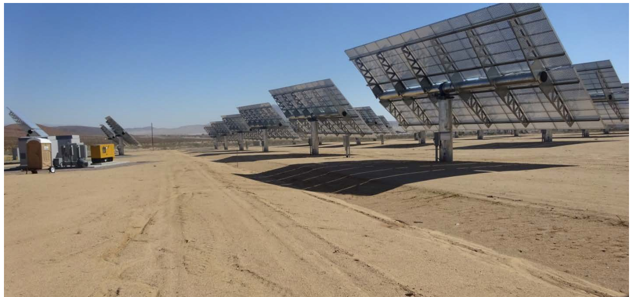
Figure 2 Plant view from the west side. The ground cover is small compacted sand/aggregate (1-2 mm size). The site slopes downward from west to east and includes the drainage ditch shown paralleling one row of trackers.
