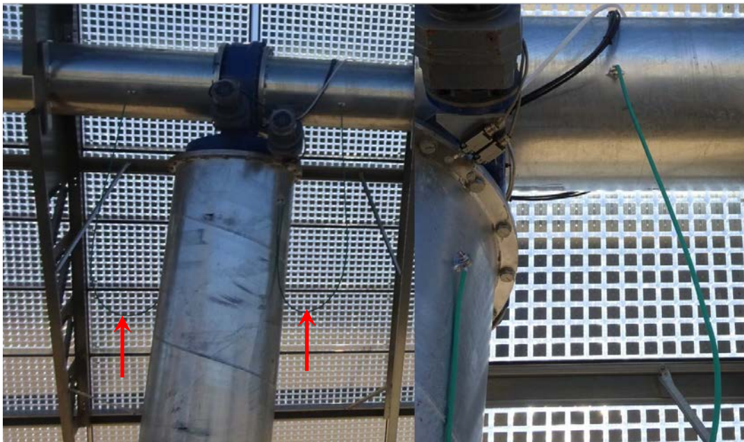
Figure 10. (Left) Red arrows point to grounding wires that connect the tracker pedestal to the left and right horizontal yoke tube that supports the array structural ribs. Although not shown here it was verified that each CX M500 module also was grounded.
