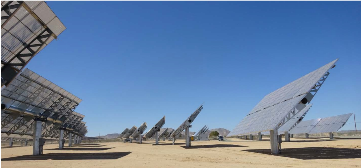
Figure 1 Plant view from the east side. All trackers were on sun throughout the inspection period.
