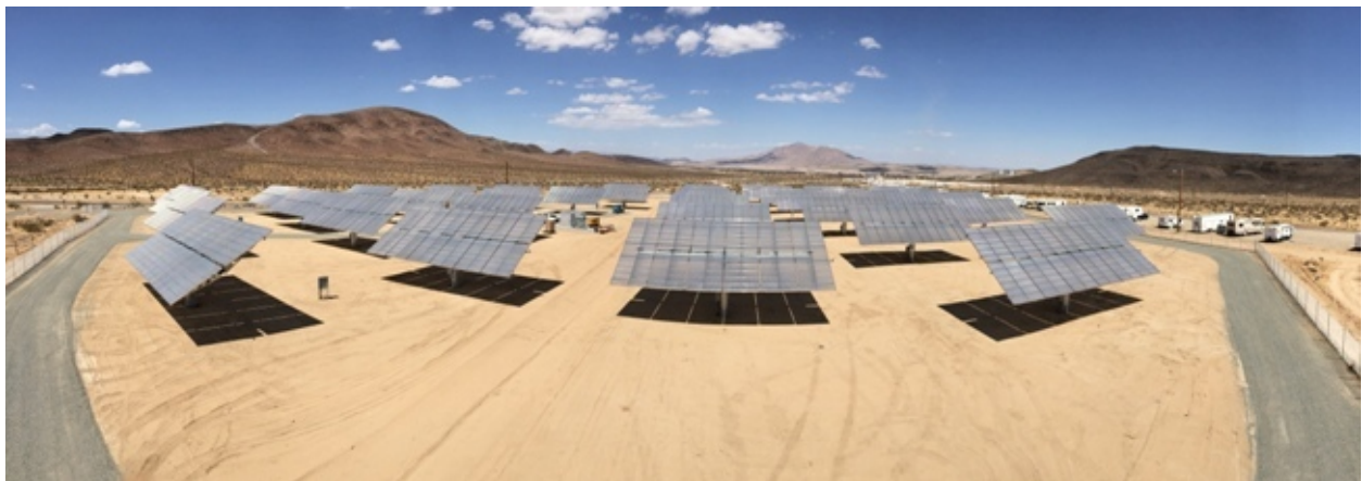
Figure 11. CPV Plant at Fort Irwin
