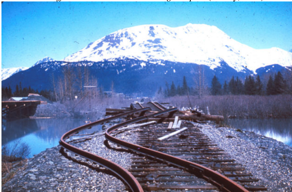
Alaska railroad rails torn from its ties (Survey, 1995)
