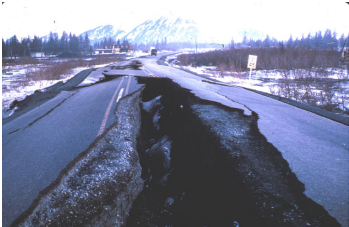
Fissures opened on highway near Portage, AK (Survey, 1995)
