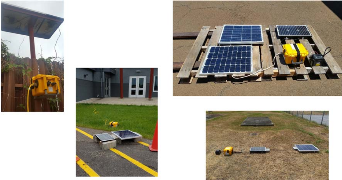
Figure 3.3: Installed Test Systems
