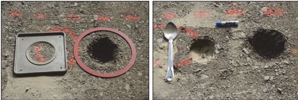
Figure 31. Example of sand cone versus photogrammetry holes. Note the photogrammetry technique is more conducive to a larger excavation
