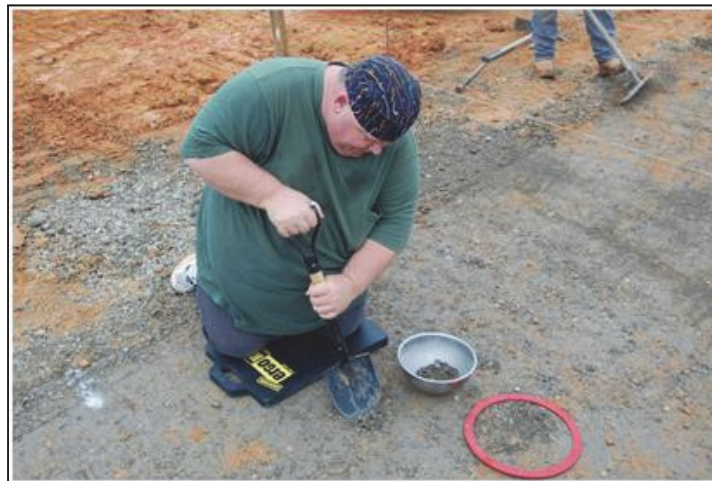
Figure 2. Using a shovel to excavate soil at a location where soil density is required. Note bowl to store soil in and red ring for calibrating distance.
