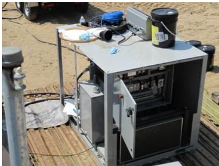
Figure 12. View of Hydraulic Power Unit (HPU).
