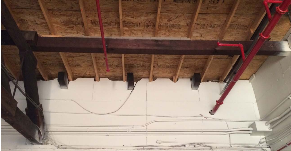
Figure 7. Photo Showing Large Holes in Wallboard at the Roof Rafters of Building M/608A at NSA Mechanicsburg
