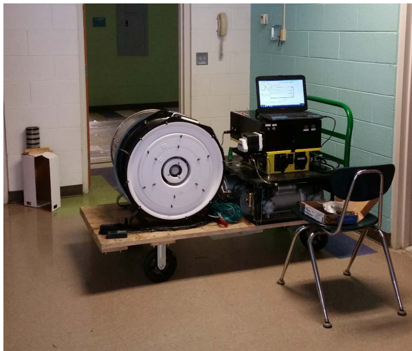
Figure 2. Photo of Aerosol Sealing Equipment Setup
