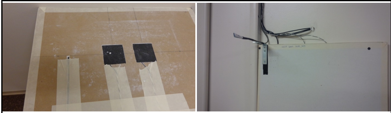
Figure 11. Photographs of a Set of Installed Heat Flux Transducer (HFT) and Temperature/Relative Humidity (T/RH) Sensors.
