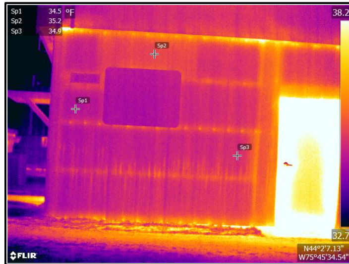
Figure 69. Failed Panels above Sign (South Face).
