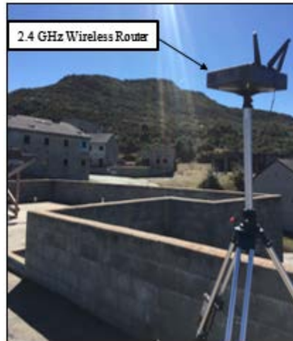
Figure 16. 2.4 GHz Wireless Router
