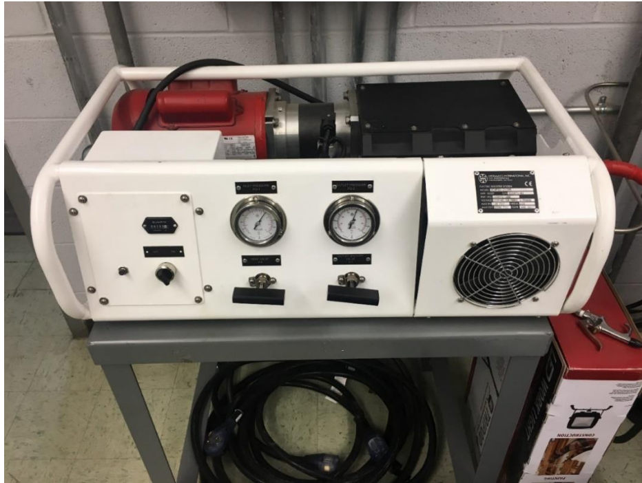
Figure 8. Primary Air Compressor
