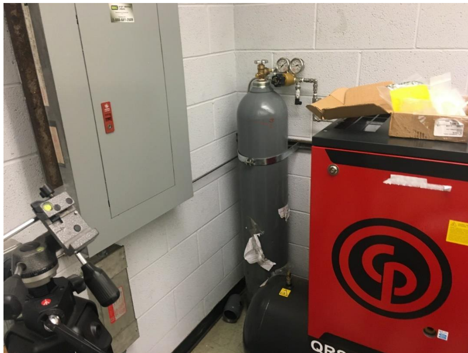
Figure 9. Compressed Air Tank
