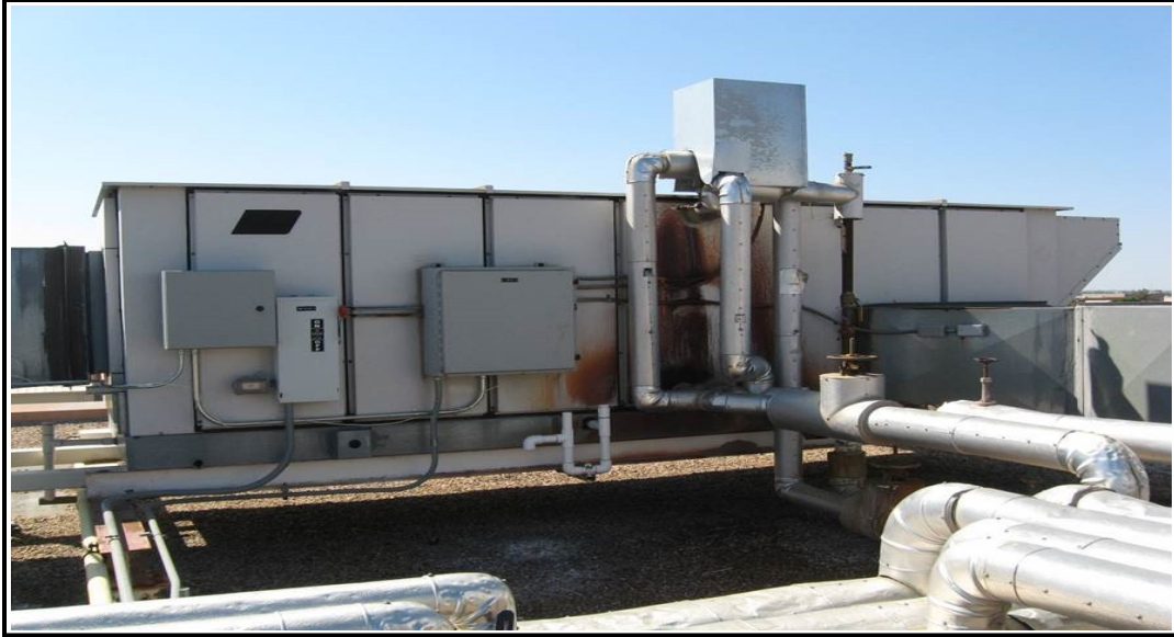
Figure 10. Existing AHU that was replaced on Bldg. 3 at Tinker AFB.
