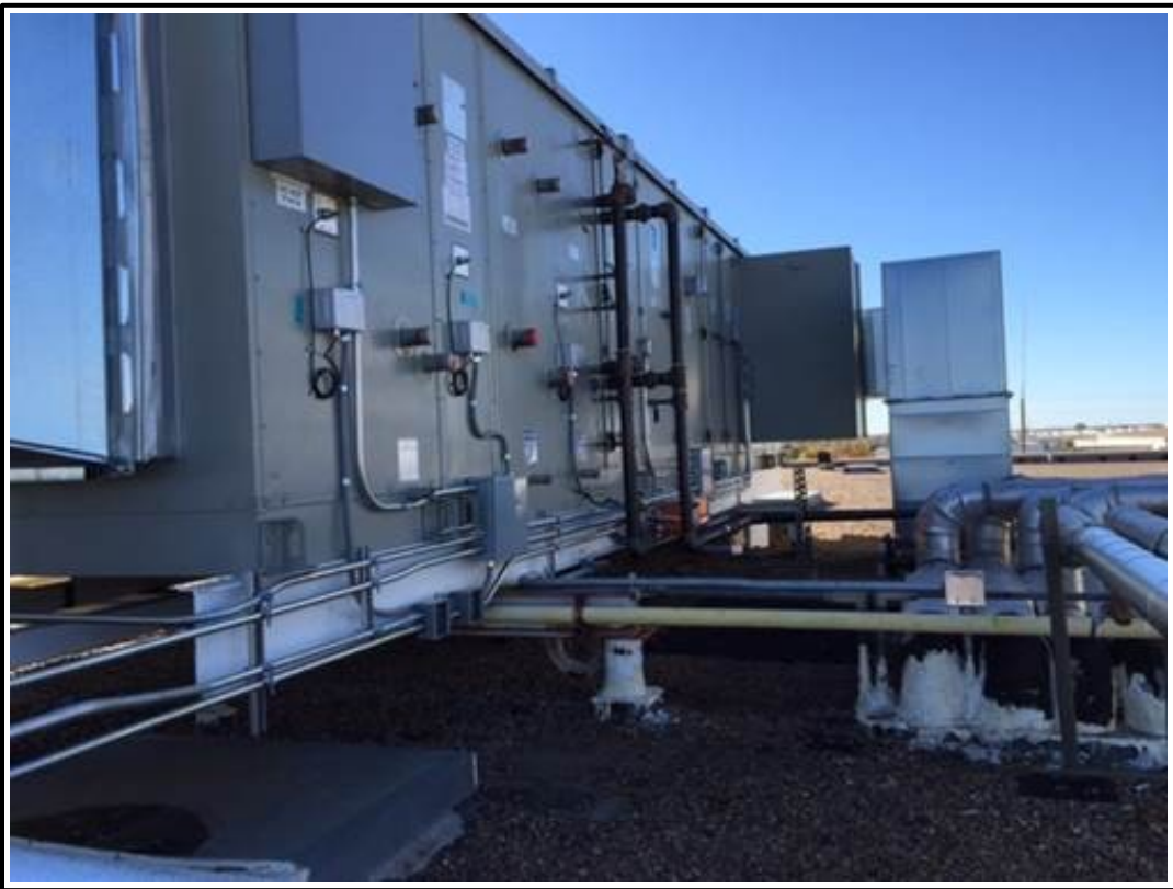
Figure 11. New HEDS AHU on Bldg. 3 at Tinker AFB.
