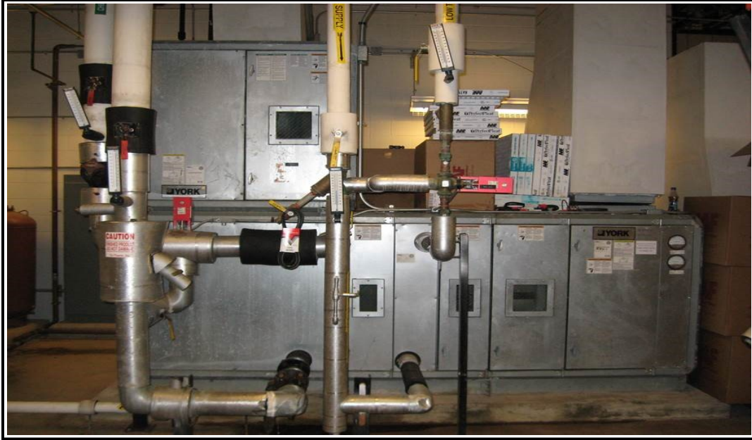
Figure 12. Existing AHU that was replaced in Bldg. A-3556 at Fort Bragg.
