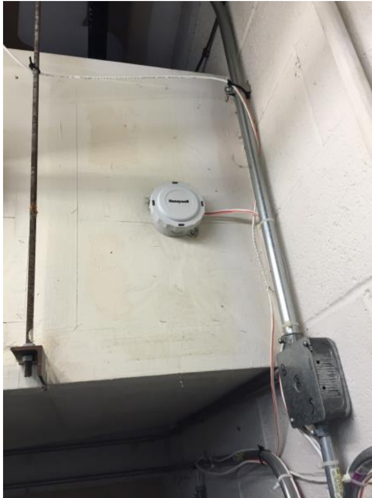
Figure 5-22. Outside air temperature sensor.
