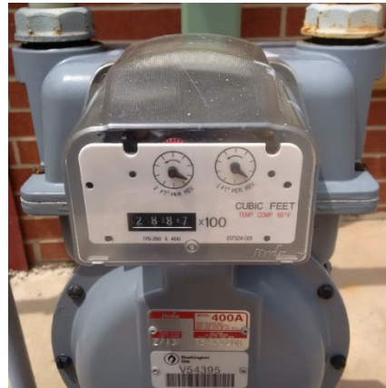
Figure 5-5. Existing utility gas meter for Bldg 1540A.
