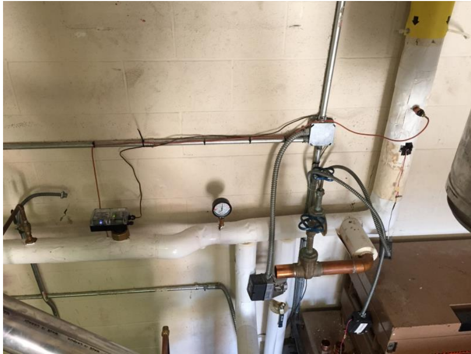
Figure 5-15. Boiler BTU Meter as installed.
