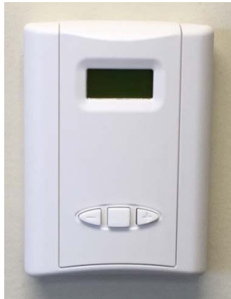
Figure 5-4. Typical room thermostat and RH sensor.
