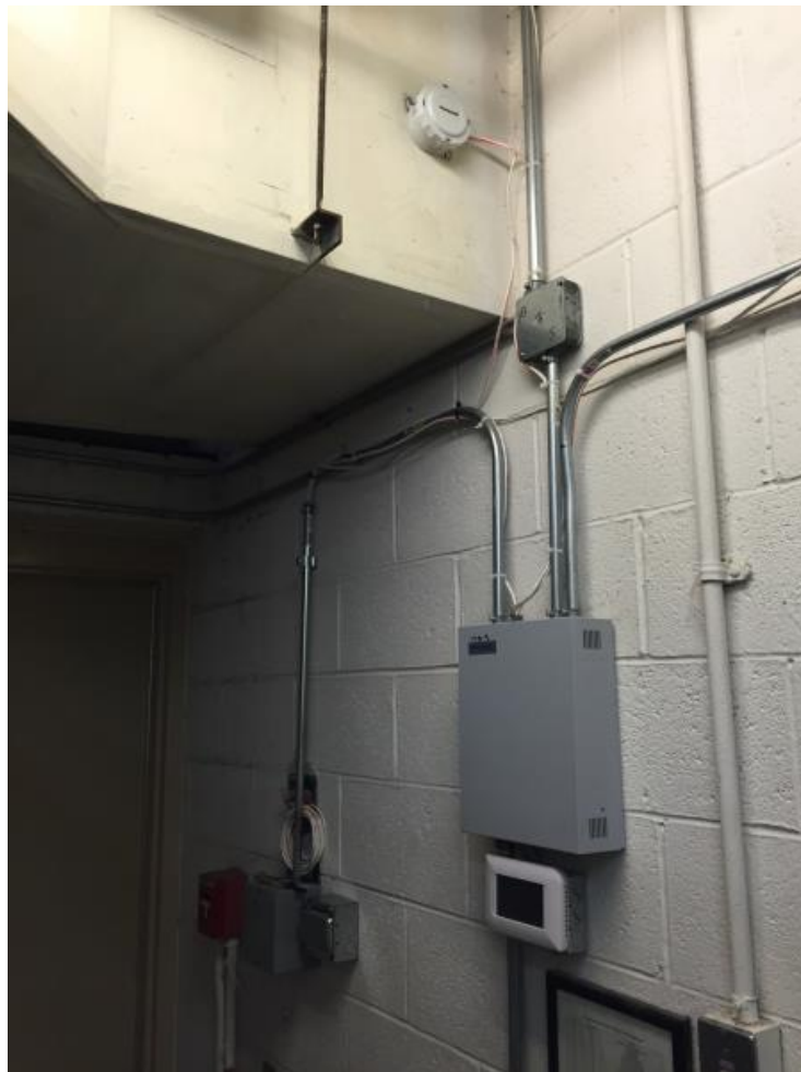
Figure 5-20. EMS installation within Bldg 1540B Mechanical Room, showing EMS controller and outside air (OA) temperature sensor.
