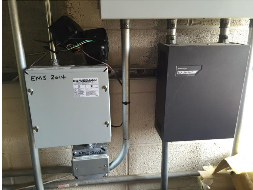
Figure 5-13. EMS panel with monitoring devices installed.
