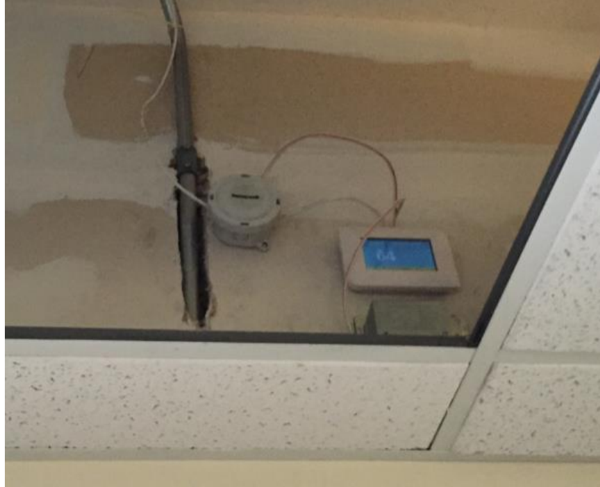
Figure 5-17. Building Envelope DP Sensor (high side inside room, low side outside building) and Wall temperature/RH sensor installed above office C003.
