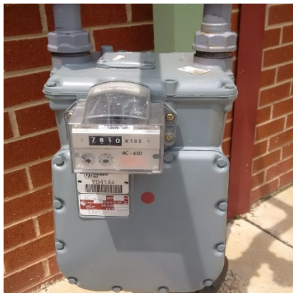
Figure 5-6. Existing utility gas meter for Bldg 1540B.
