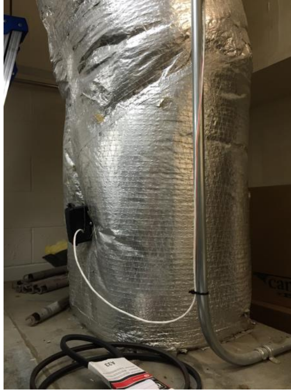
Figure 5-23. Supply air temperature AHU-4 duct sensor.
