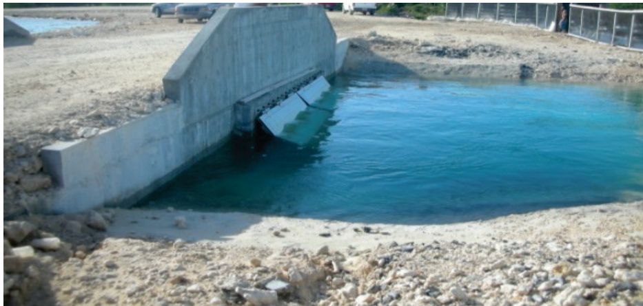
Figure 1. Example of flap gate culverts. (This photo was taken from Google Images).
