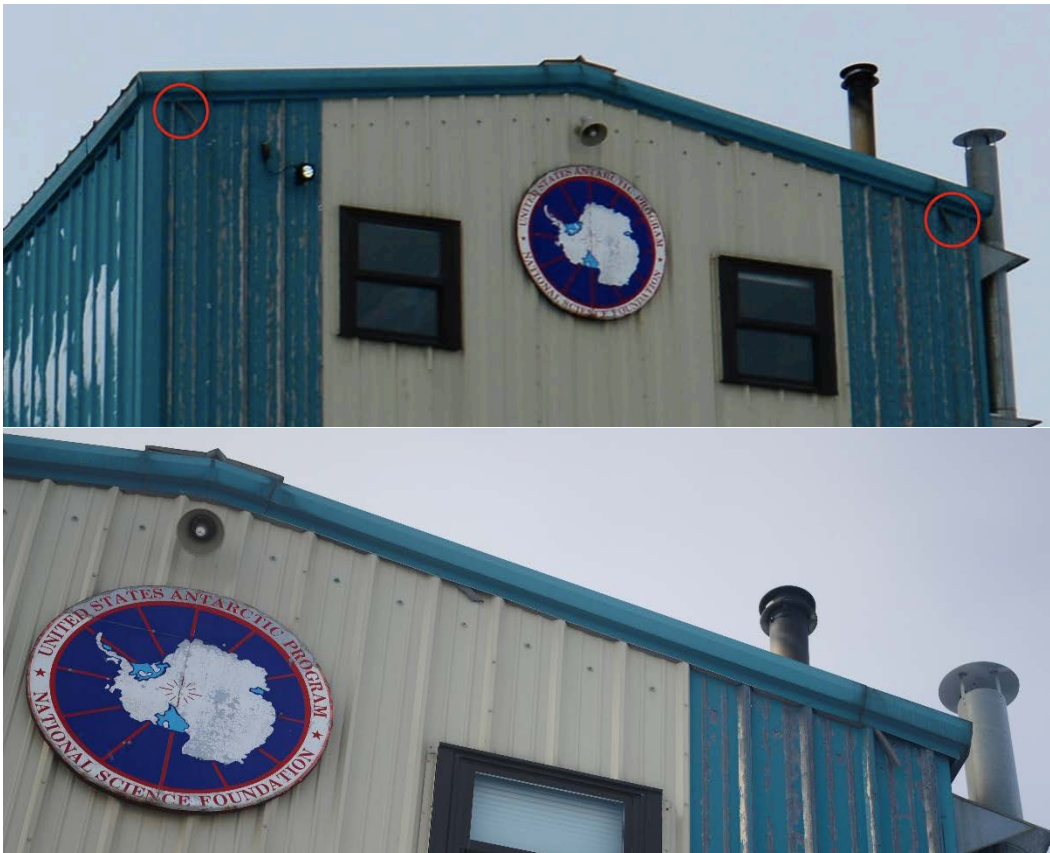
Figure 11. Detail of damaged or unseated insulation along southwest roofline soffits on the Biolab. Multiple areas were completely devoid of this insulation material.
