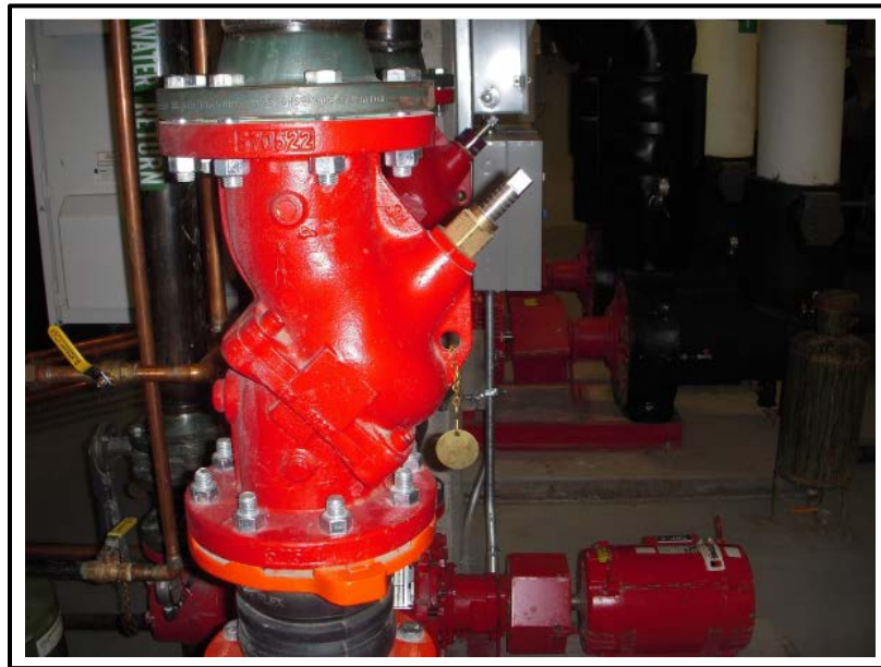
Figure 19. Pump discharge valves offer clues into oversized equipment opportunities.
