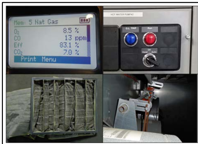
Figure 24. Test unit efficiencies, note overrides, discuss replacements, and identify failed parts.
