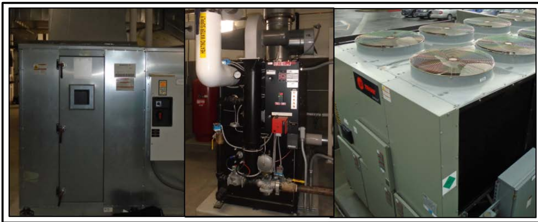
Figure 18. Air-side, heating, and cooling systems may be good candidates for no-load disables.
