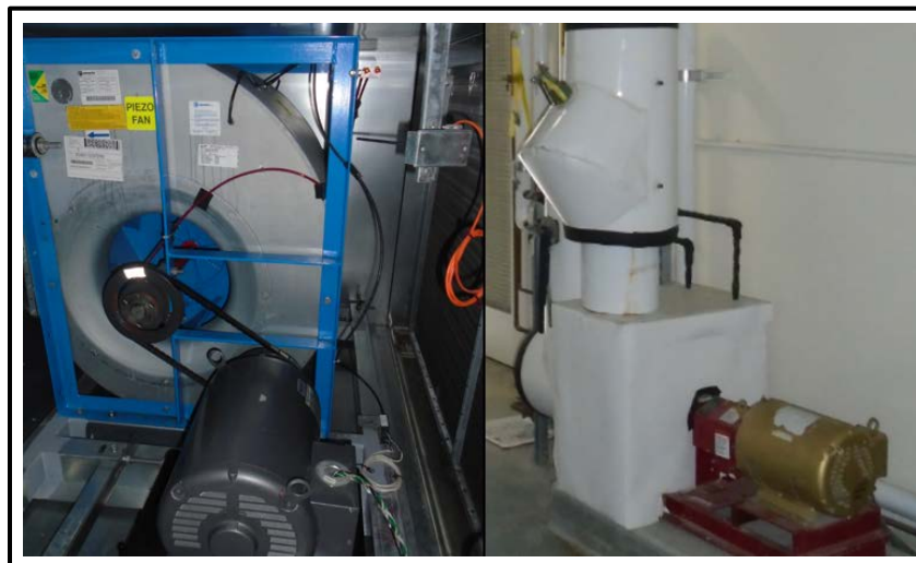
Figure 21. Most fan and pump motor systems can be readily retrofit for VFD applications.
