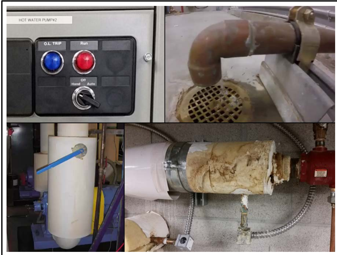
Figure 13. Examples of obvious indicators of performance: an Hand-Off-Auto (HOA) switch in hand mode may be accidental or indicative of a greater problem (top-left); active condensate drain may indicate unnecessary cooling (top-right); throttled pump discharge valve could mean oversized equipment (bottom-left); improperly installed sensors may be misleading control systems (bottom-right).
