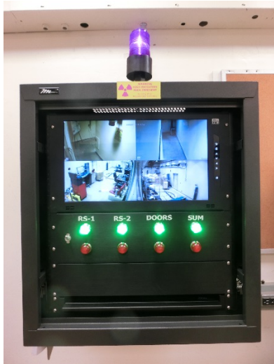
(a) Interlock Control Panel
