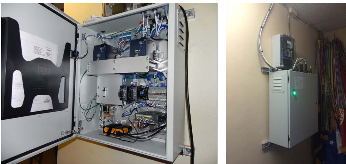
Figure 12. Control Panel (with power supply and network controller) Installed
