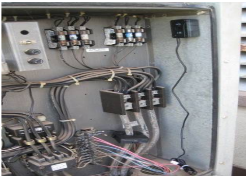
Figure 14. Chiller Power Measurement
