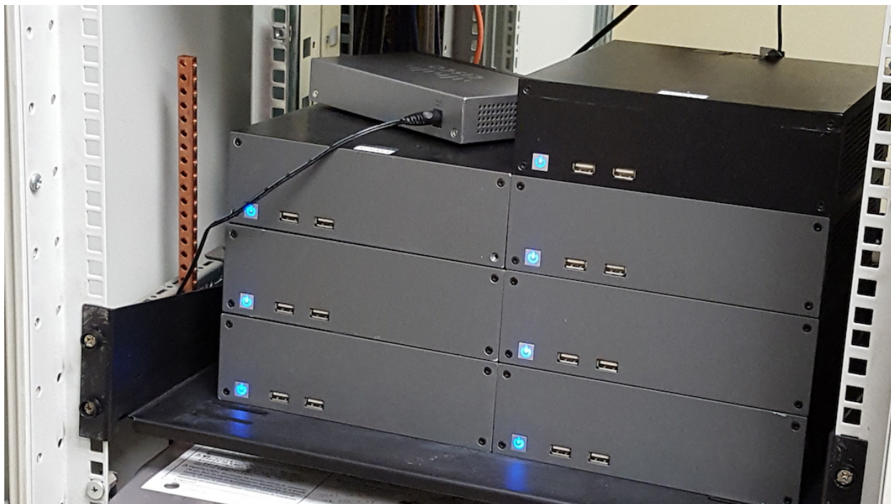
Figure 16. Spire and Switch in a Rack In the Power Plant (4U high)
