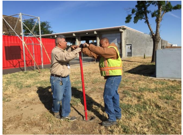
Figure 7. Isolating Valves Up- and Down-Stream
