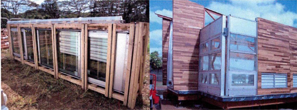
Figure 4.5.8 Crated curtain wall components at Ilima (l) and installed curtain wall at Kawaikini (r)
