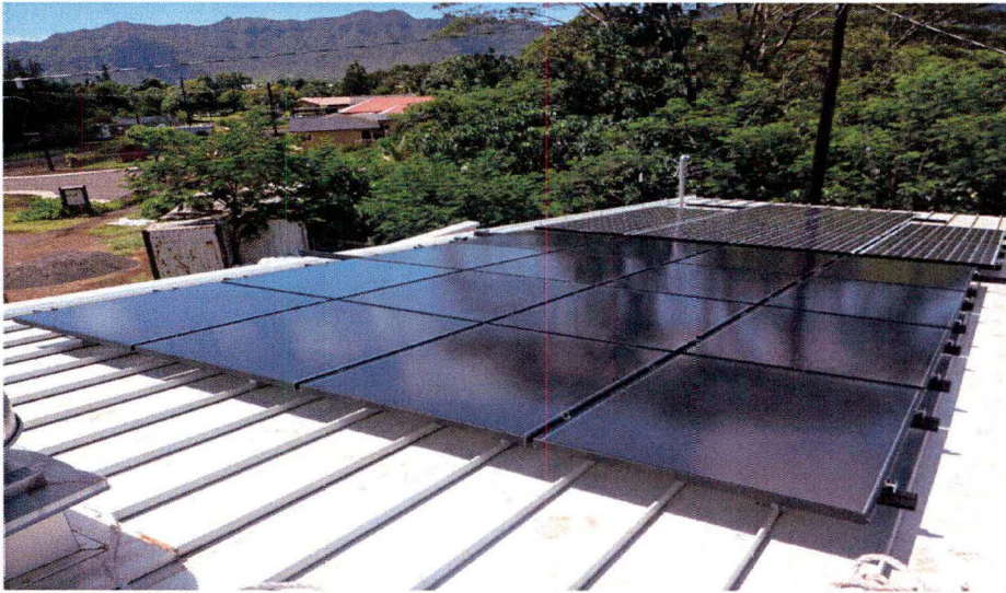
Figure 3. Kawaikini East classroom, East Kauai, showing two PV systems both connected in string configuration, CIGS (top) and monocrystalline (bottom).
