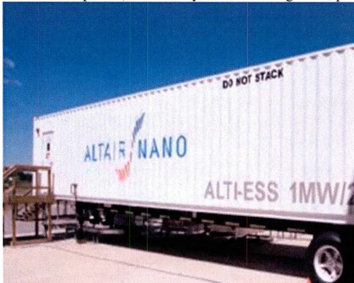
Figure 4.2.1: Power Module (PM) houses batteries as well as other systems.
