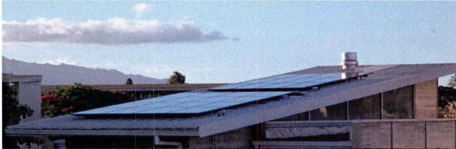
Figure 1. Ilima classroom, South Oahu showing the two PV systems installed to compare heterojunction with intrinsic thin layer (HIT) to thin film made of copper, indium, Gallium and diselenide (CIGS), both in a string configuration. HIT is located on top and CIGS at the bottom.
