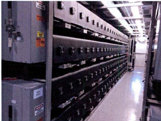
Figure 4.2.12: Interior of the power module (PM).
