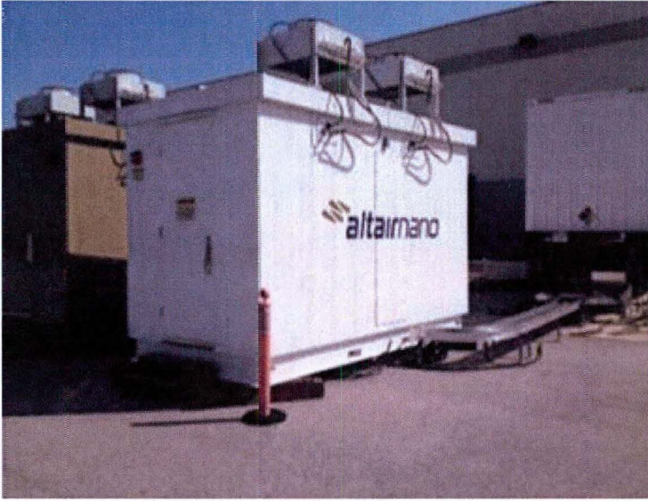
Figure 4.2.2: Power Conversion System (PCS) contains inverters and all necessary support systems.
