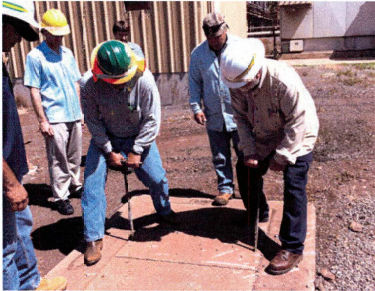
Figure 4.2.10: Initial site visit to main Molokai power station. Workers provide access to underground conduits.
