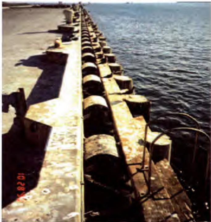
Photo 3. Pier Bravo. Existing treated timber fender system on the outboard side of the main pier.
