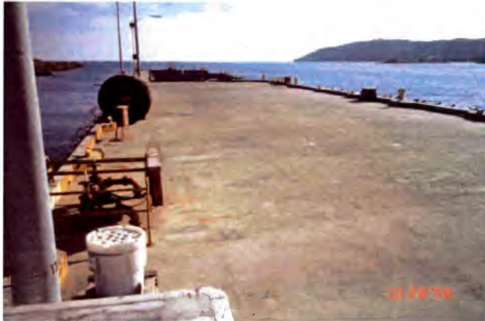
Photo 1. Pier Bravo. Overview of the south half of the main pier and the southern extension.
