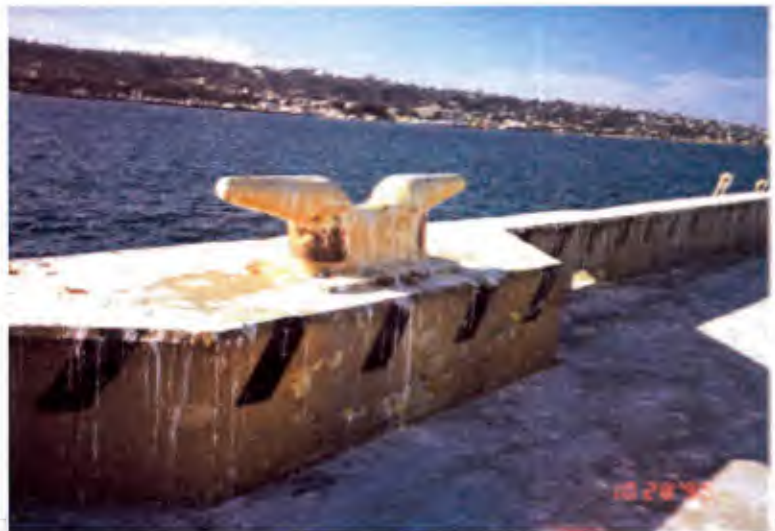
Photo 8. Pier Bravo. Concrete delamination at the side of a mooring cleat on the main pier.
