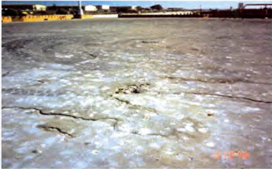
Photo 5. Pier Bravo. The existing concrete deck surface has extensive delamination at nearly 100% of the previous partial repair areas. Delamination of the deck quickly leads to open surface spalls which impede forklift traffic on the pier.
