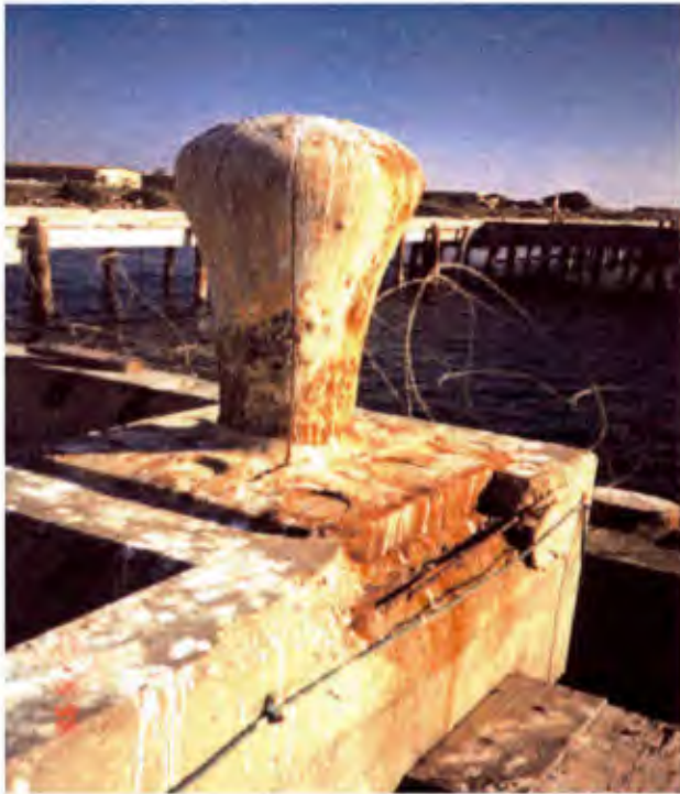
Photo 7. Pier Bravo. Concrete curb spall at a mooring bollard on the main pier.
