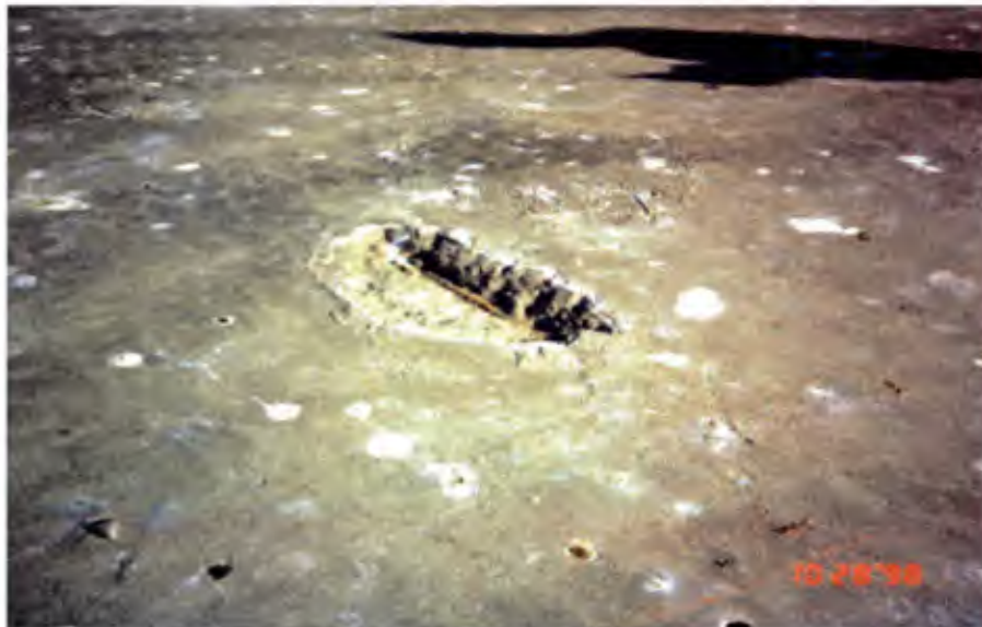
Photo 6. Pier Bravo. Delamination and surface spalls are caused by corrosion of steel reinforcing bars in the concrete deck. The past use of seawater to clean the deck is most likely responsible for the rapid decay of this deck.
