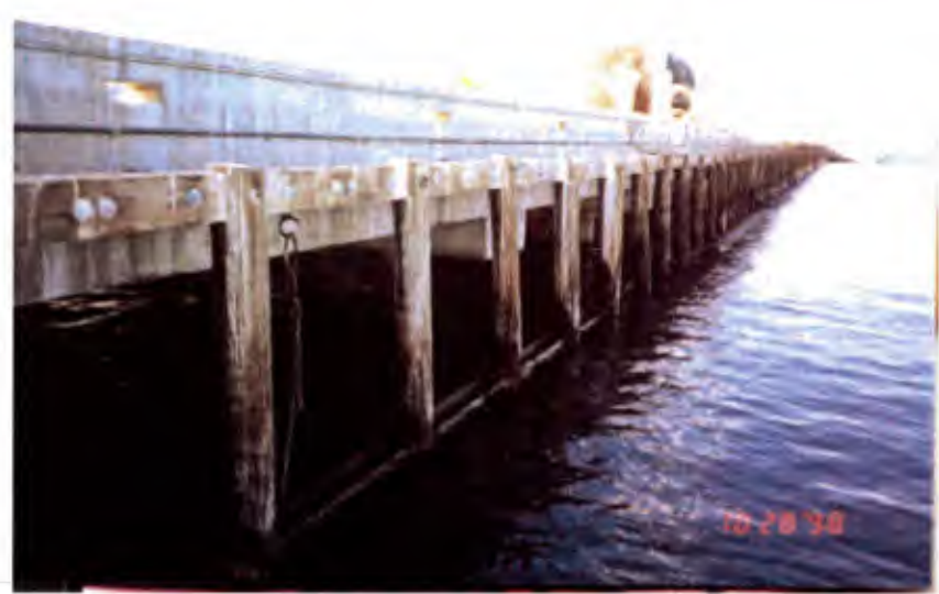
Photo 4. Pier Bravo. Existing treated timber system on the inboard side of the main pier.
