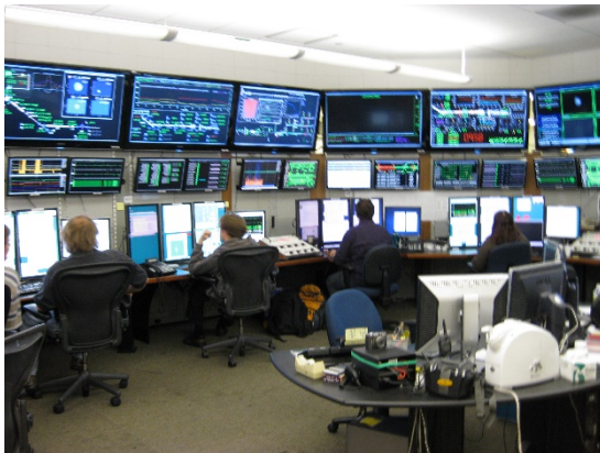
Primary Control Room
